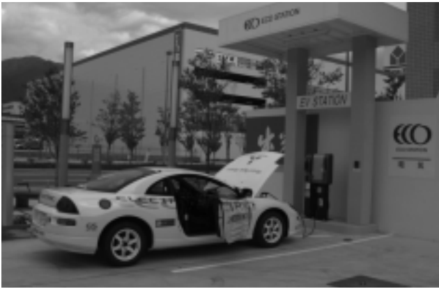
Fig. 5 Commercial EV charging station in Kobe
