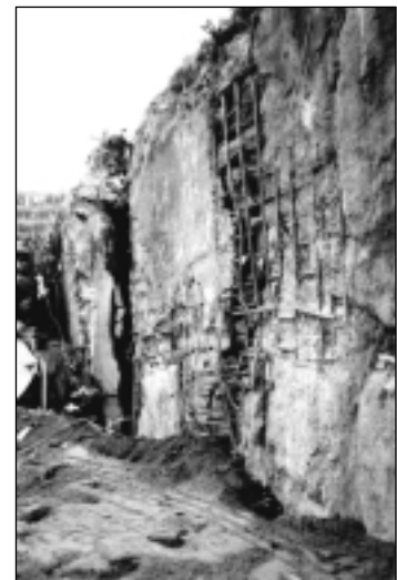
FIGURE 12 Damaged walls at Greenwich Street.
