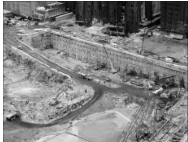
FIGURE 11 Progress along the Liberty Street slurry wall showing the installation of the fourth-tier anchors.
