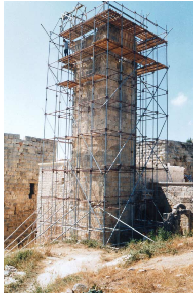
section was carefully taken apart and largely rebuilt, using new stones where the original were beyond repair.
