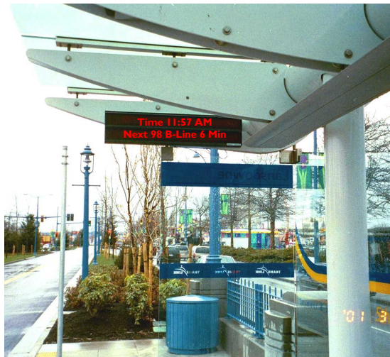
Exhibit 2.3.3: Passenger Information DMS at Stations
