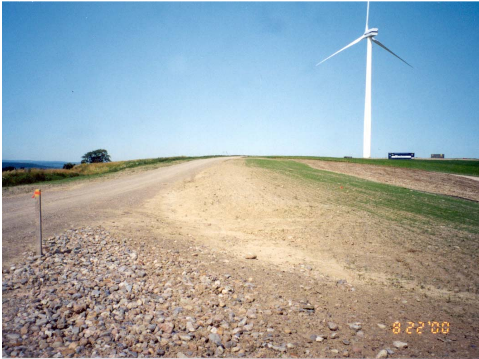
Seeding failed along the access road due to a lack of topsoil. Imported topsoil is needed to correct areas such as this.
