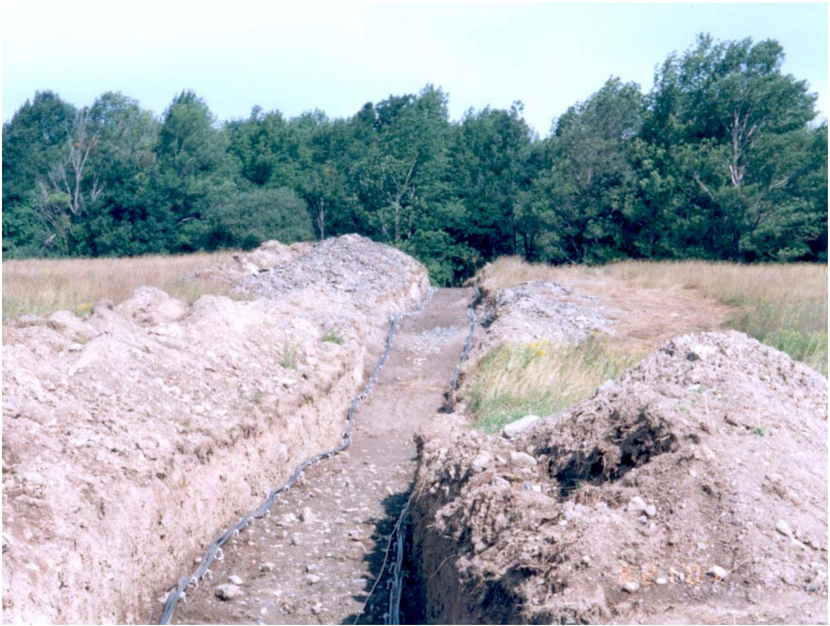
Trenches excavated for the collector system can cause significant impact to farm fields. This photo shows poor separation of topsoil and subsoil.
