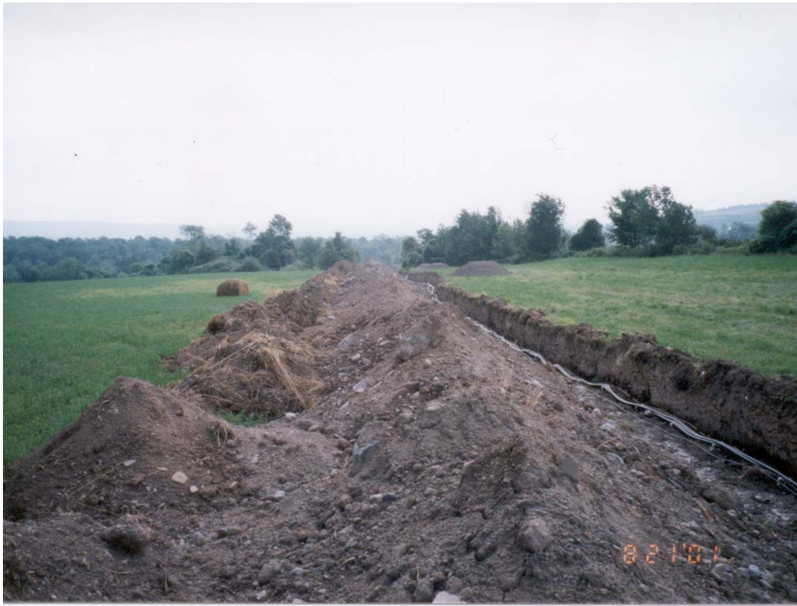
The contractor attempted to separate the topsoil (left side) from the subsoil material (right side). Some mixing did occur because of limited work space.
