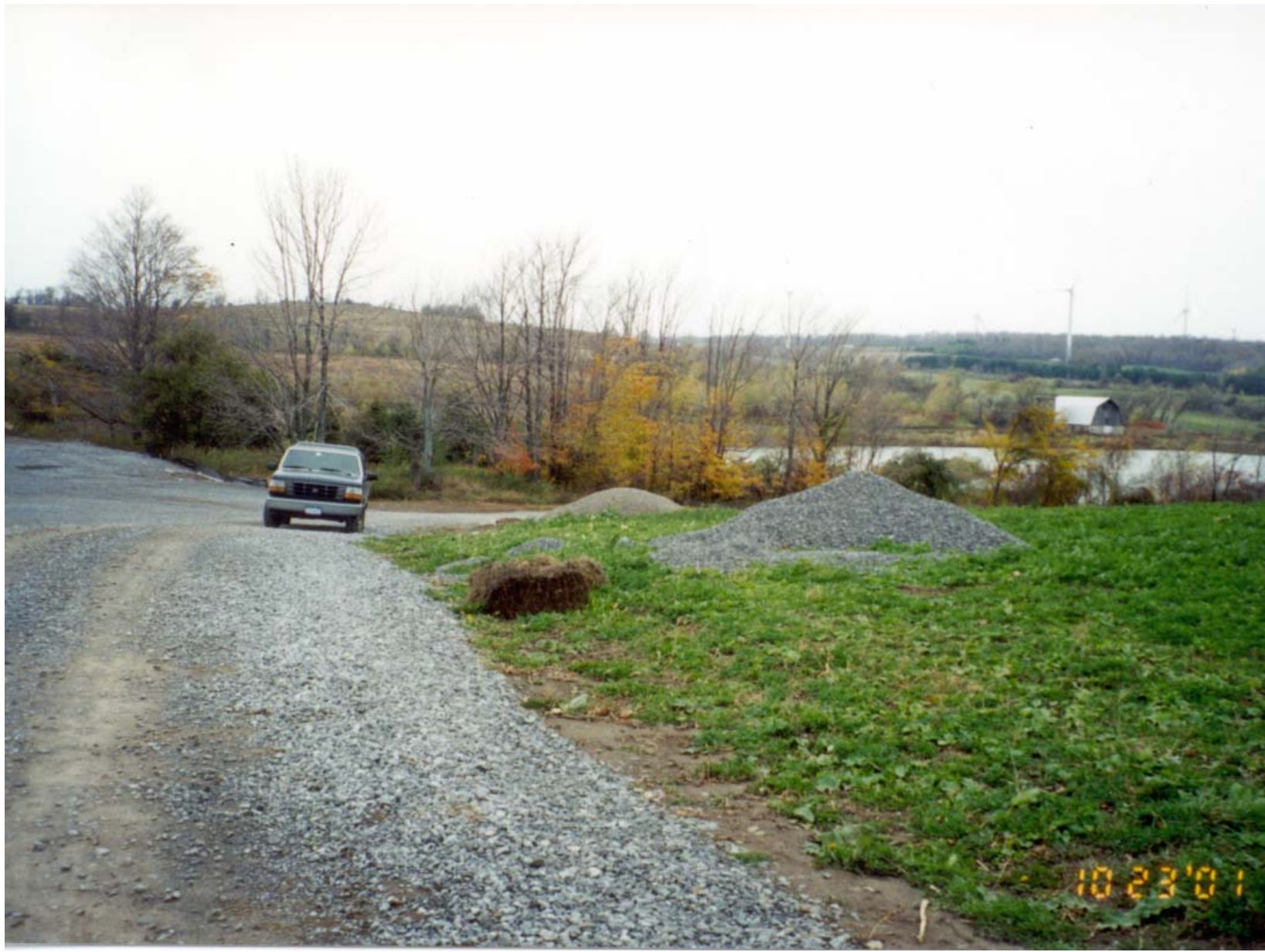
Crushed stone should not have been dumped in the agricultural field. Some stone was left in the field after restoration causing damage to the alfalfa stand.
