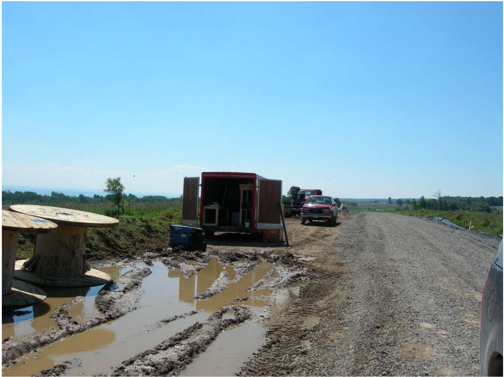
Topsoil stripped from area adjacent to access road to prevent damage as a result of vehicle traffic and parking.
