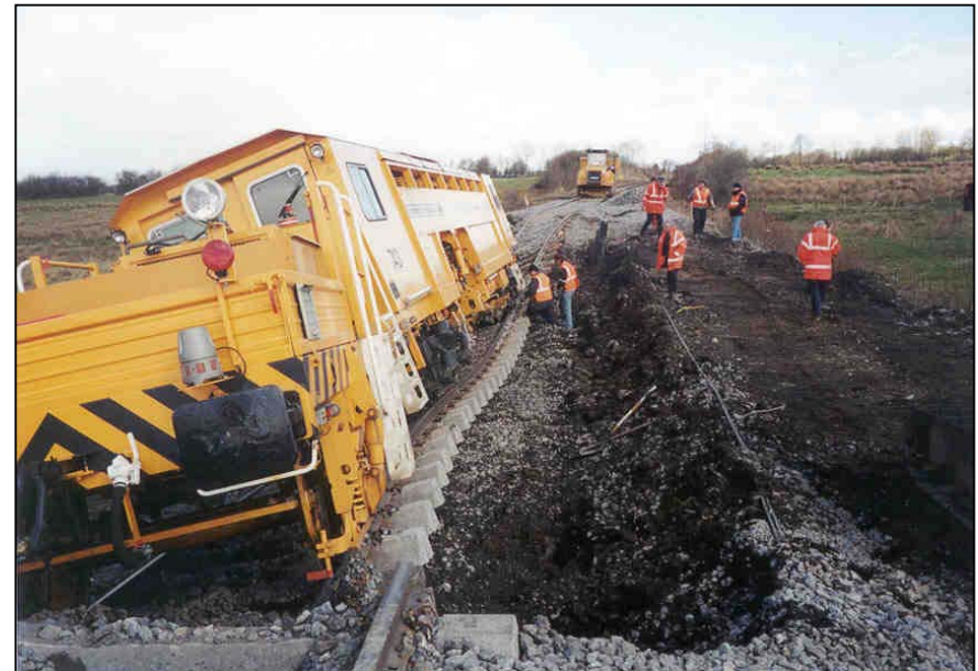
Embankment failure on the Sligo line near Ballymoate 2001.
