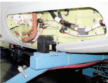
The view through an access panel under the pilot station of electrical, heating and control systems.
