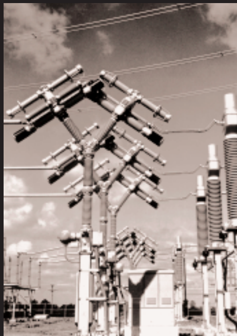
Installation de couplage haute tension, 1974
