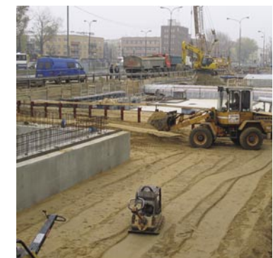
The construction status of the first line – B20 section – A23 – the Młociny junction (the status for 15.06.2006).
