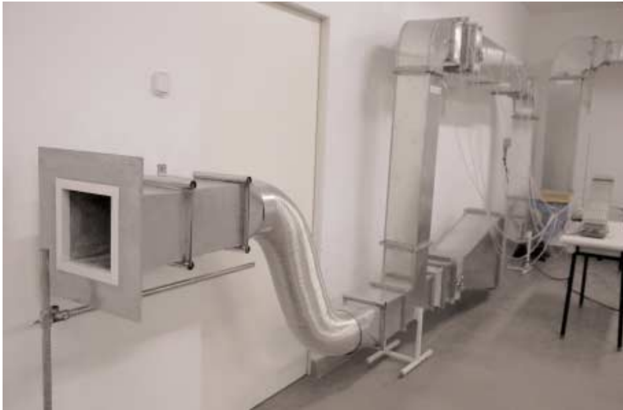
Laboratory of ventilation
