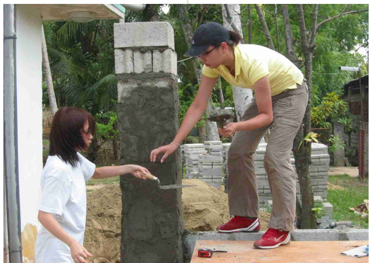
The team worked hand in hand to rebuild the villagers' homes and a school in Galle.
