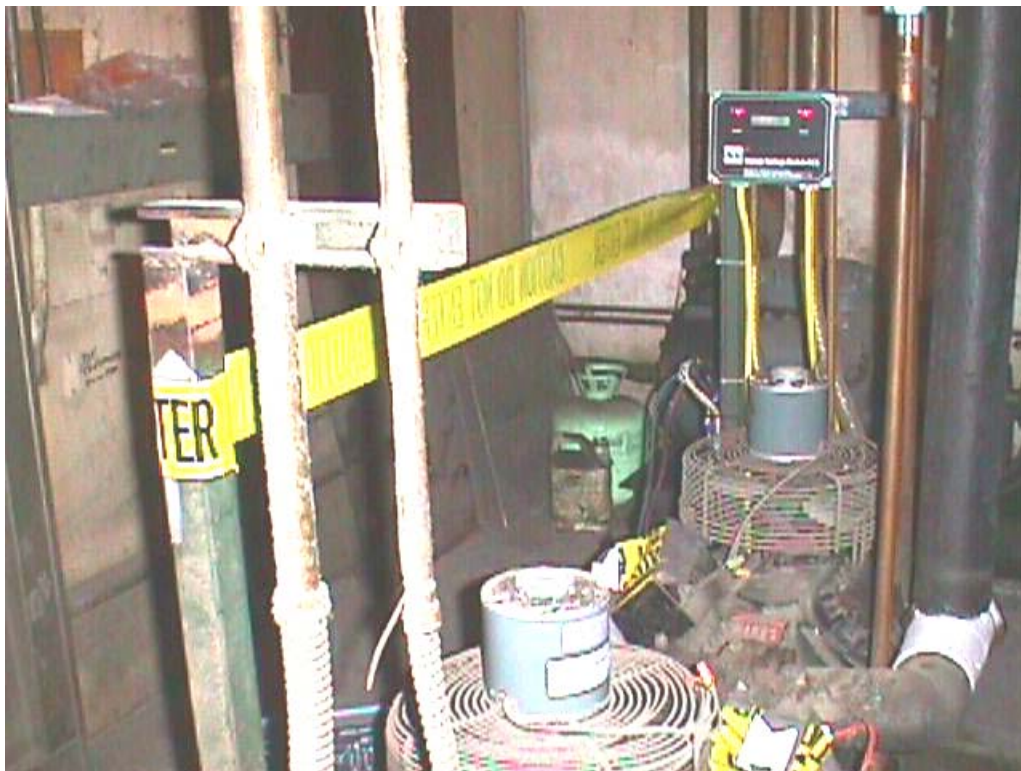
Energy Saving Module EC2 installed on compressors
