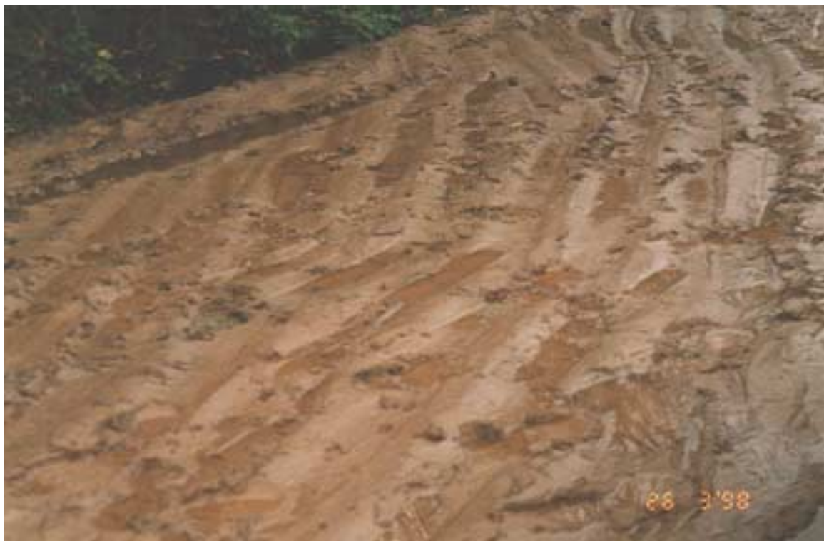
Fig 4.2: Failure of cuttings to compact resulting in unstable, water logged surface
