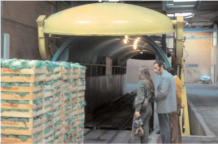
Figure 57: Vacuum cooling. Both cooler ends are lifted to allow moving produce in and then closed to create a vacuum.
