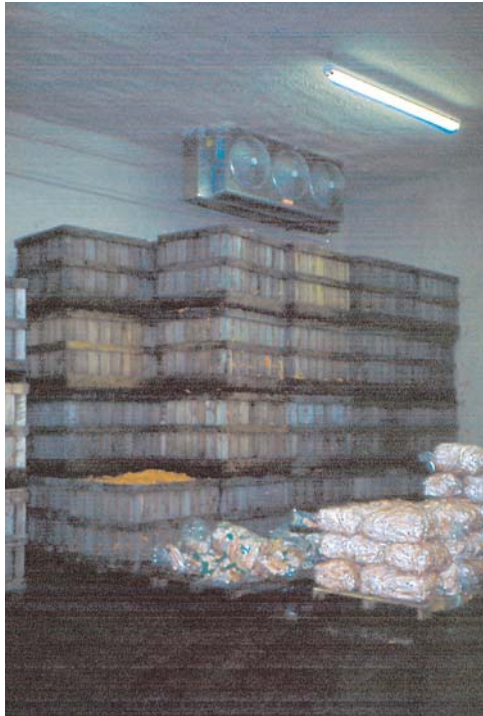
Figure 53: Inside refrigerated storage. Evaporator is located on the upper part of one of the walls.
