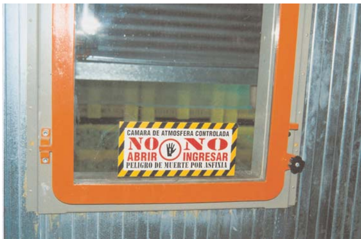
Figure 60: Inspection window in a room with controlled atmosphere.
