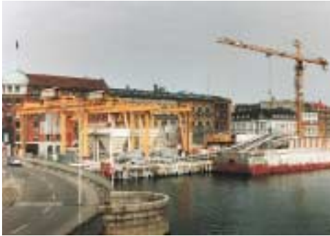
The former main construction site in Havnegade where limestone and soil spoil was excavated and new tunnel sections were lowered onto the work train.
