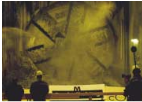
From the breakthrough of a tunnel drill into a tunnel station. The tunnel drill bores a hole 5.5 metres in diameter.
