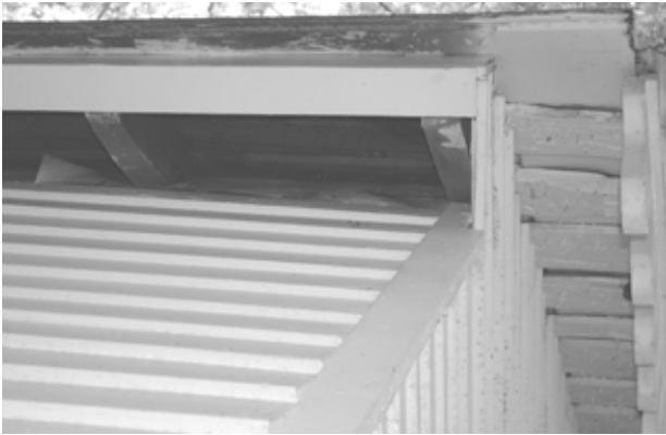
FIGURE 52. View of northwest corner of house, showing typical roof decking and exterior finishes. (T. Jones, NPS, 2004)
