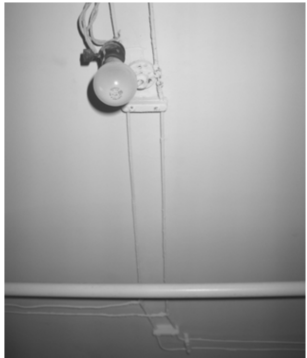
FIGURE 69. View of a portion of the knob-and-tube wiring system, which is no longer active. (T. Jones, NPS, 2004)
