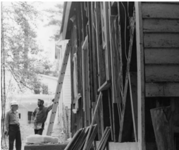
FIGURE 41. Chief of Maintenance Charlie Hamm, left, and Joe Moore, temporary carpenter, at front of house with siding removed, 1977. (CARL4008/03/38P)
