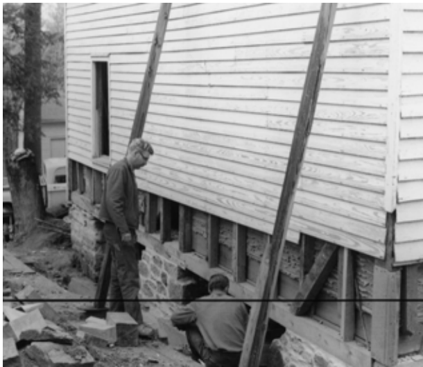
FIGURE 40. Glenn Barnwell, former maintenance employee, standing, inspecting foundation repairs at rear of house, 1977. (CARL4008/03/27P)
