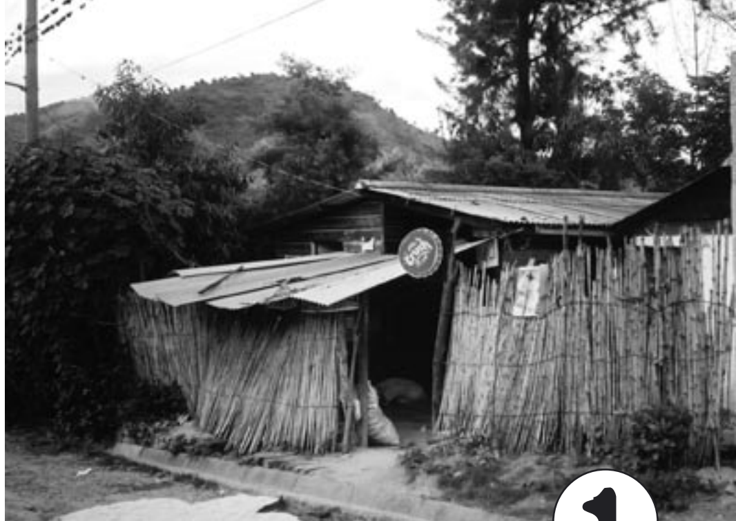
Inadequate housing at the Pacux resettlement site
