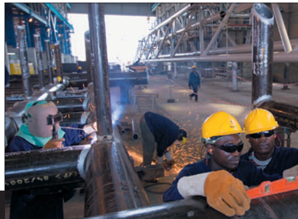
Fabrication for the Erha development is under way in Port Harcourt, Nigeria.
