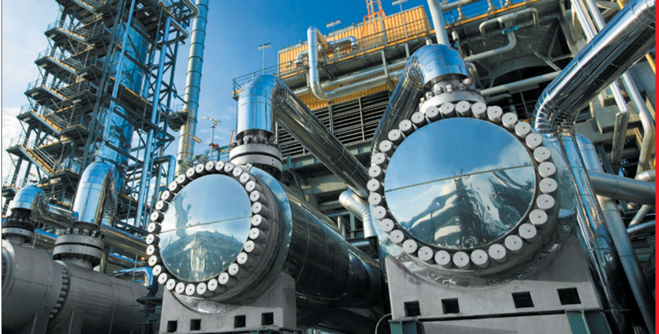
ExxonMobil's new GO-fin ing Unit and related facilities at Port Jerome-Gravenchon, France, increase the yield of lower-sulfur motor fuels and high-value chemical feedstocks.
