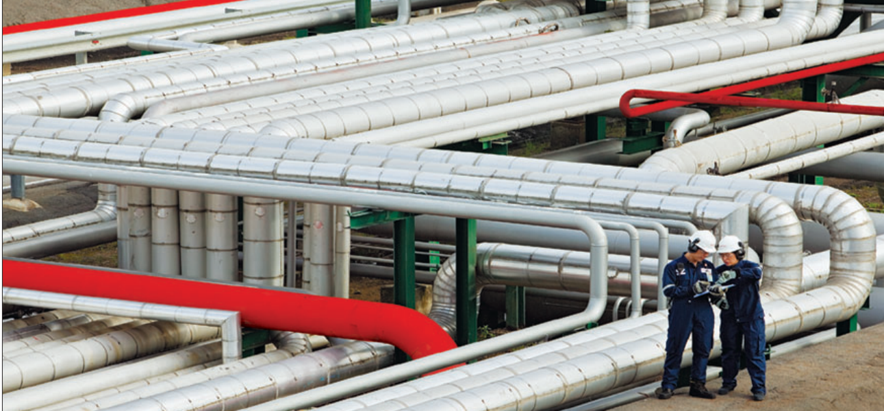
At our largest petrochemical complexes, more than 60 products are transferred between the refinery and the chemical plants.
