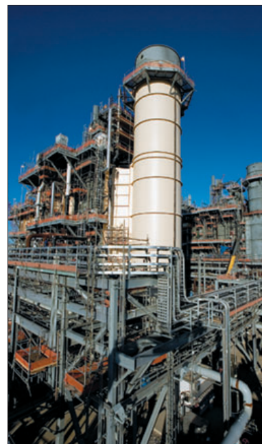
A new cogeneration facility at ExxonMobil's Beaumont, Texas, refinery improves energy efficiency and reduces emissions.
