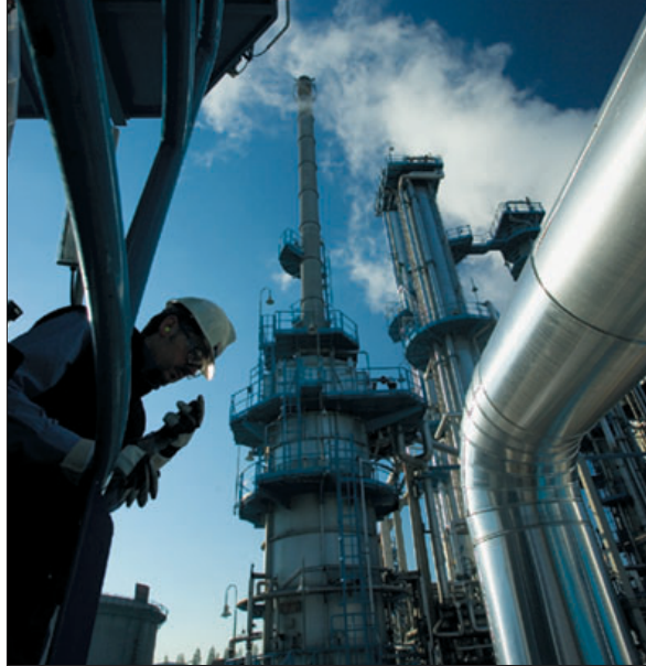
A modified Hydrofining Unit started up in 2004 at ExxonMobil’s Treccate, Italy, refinery, along with a new SCANfining Unit to efficiently produce lower-sulfur mogas and diesel with minimum investment.
