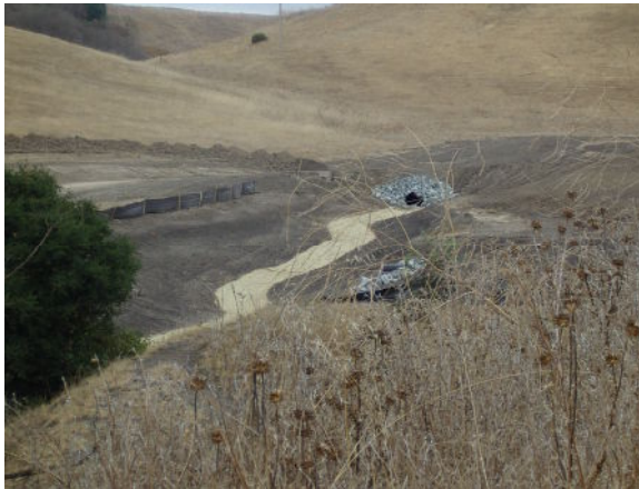
Figure 30. Erosion control efforts associated with the installation of a new equestrian facility (work in progress).
