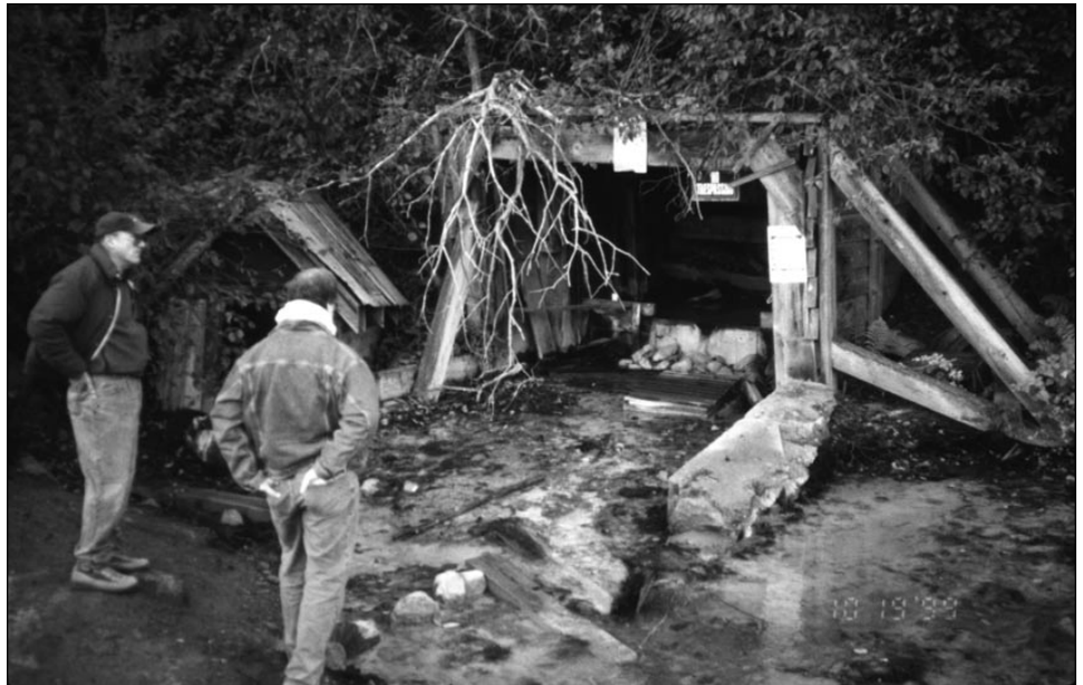
Figure 2. Mine portals and adits such as this one at the Holden Mine can be dangerous physical hazards and sources of water pollution when acid mine drainage is generated and metals are transported to surface or ground water.
