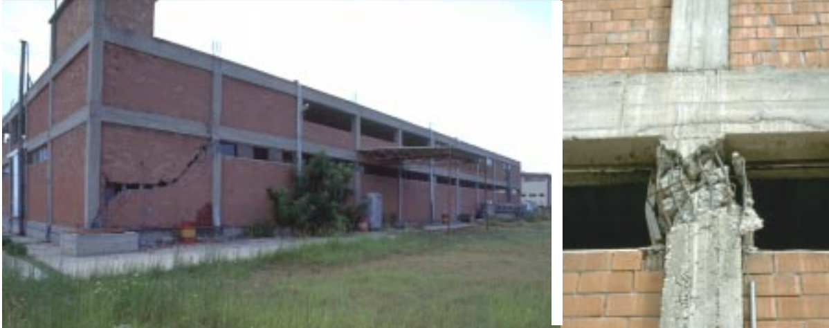
Fig. 28 Two story concrete frame building with partial masonry infill (left), detail of shear failure of reinforced concrete column by the short-column effect (right), (damage grade 3)
