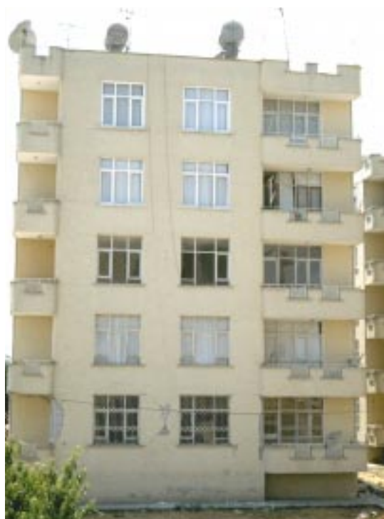
Fig. 16 With few exceptions only the damage is found in the ground floor or in the ground floor and the second floor (damage grade 2)
