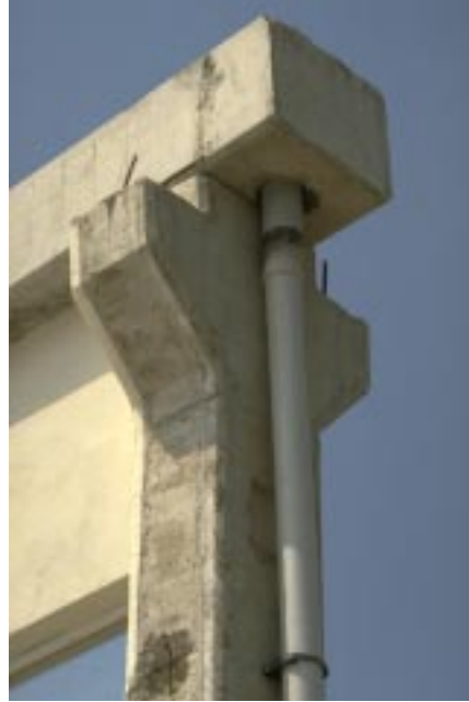
Fig. 25 Column top of precast pin-connected frame; the roof beam fell off the left column corbel
