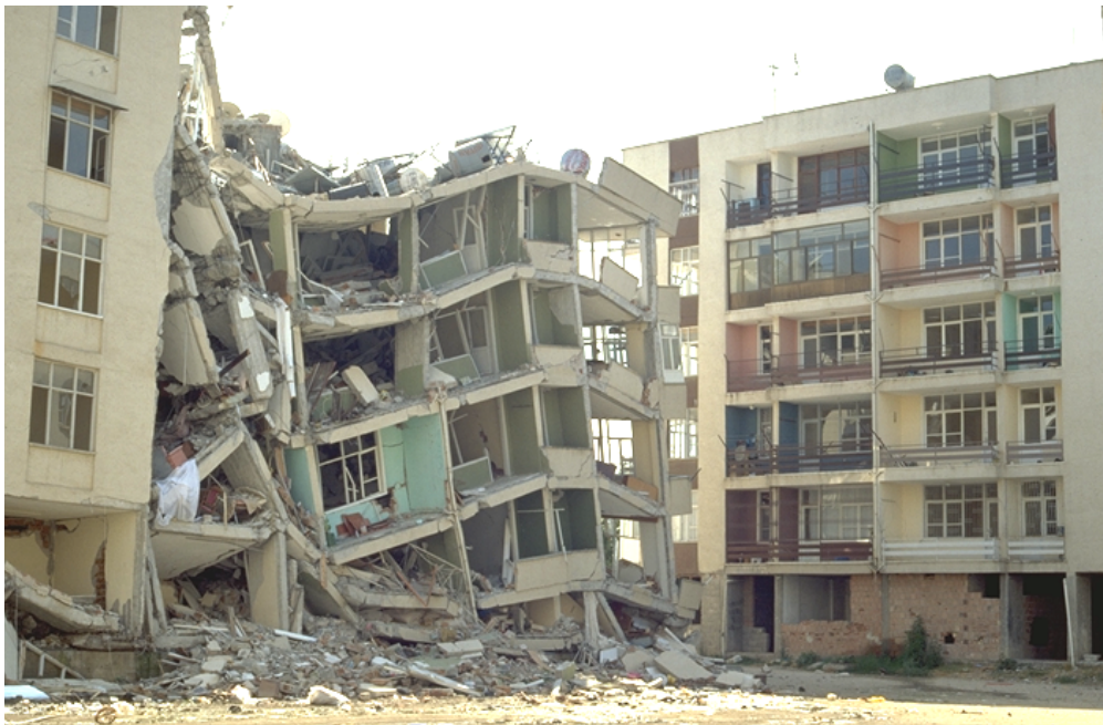
Fig. 19 Two adjacent similar buildings with very different damage pattern. The building on the left totally collapsed in the ground floor (damage grade 5) while the building on the right has slightly to moderately damaged structural walls and masonry infills (damage grade 3)
