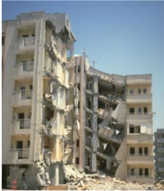
Fig. 17 Partially collapsed residential buildings in the Cumhuriyet Mahallesi district of Ceyhan; one residential building shows a partially collapsed ground floor while the upper floors remained relatively stable (damage grade 4)
