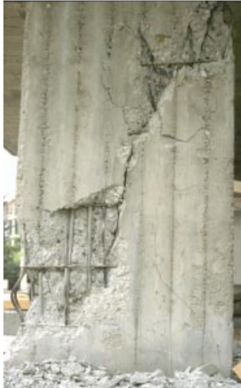
Fig. 15 Shear damage to a wall-like frame column in the ground floor of an eight-story building (damage grade 3)
