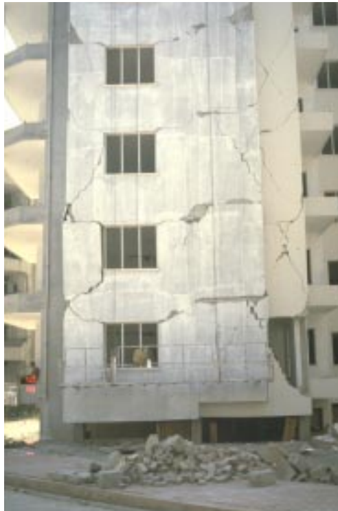
Fig. 12 Typical damage to masonry infills in the form of X-cracks (damage grade 3)
