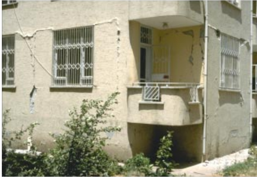
Fig. 13 Cracks between the reinforced concrete frame and the masonry infills showing the incompatible deformation behavior of the two elements (damage grade 2)
