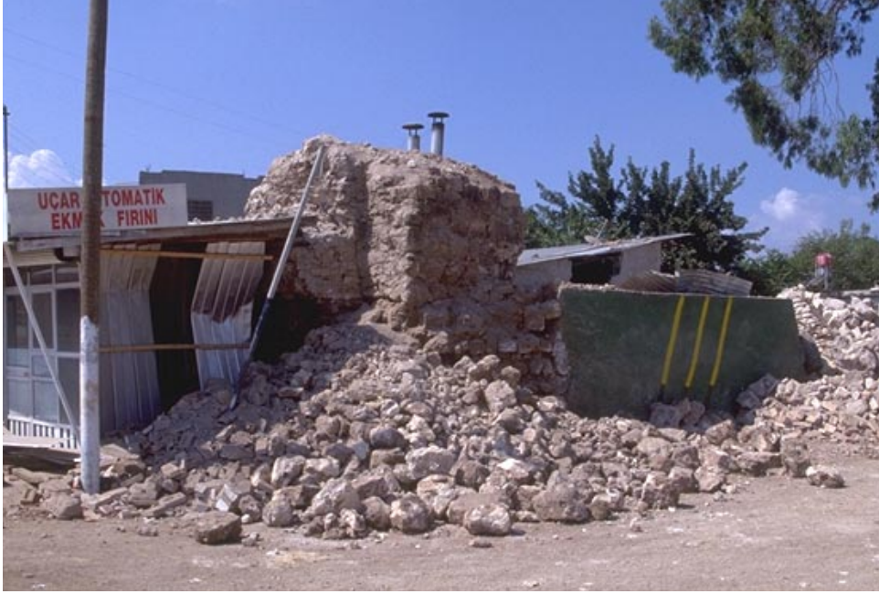
Fig. 30 Destroyed rural building made of field stone masonry in the epicentral area near Gecitli (damage grade 5)
