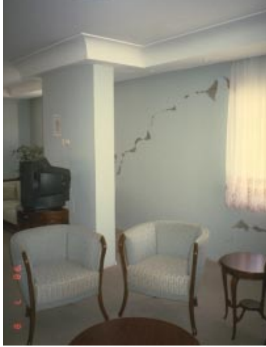
Fig. 20 Damaged masonry infill in the second story of Hotel Takav, a reinforced concrete frame building in Adana (damage grade 1)
