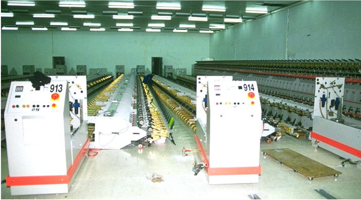
Fig. 26 Toppled spinning machines caused directly by the earthquake shaking interrupted production for several weeks
