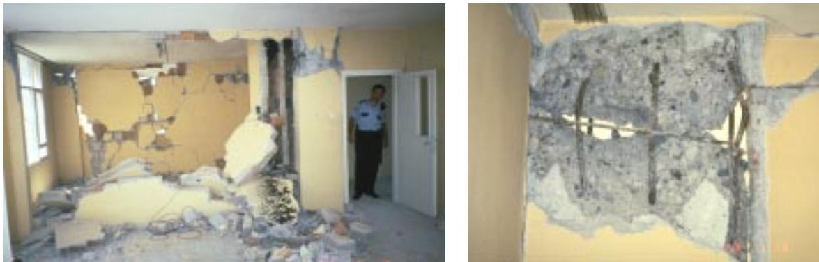
Fig. 14 Total destruction of the masonry infills by large differences between the horizontal displacements of top and bottom slabs (left), detail view of the upper part of the reinforced concrete column (right), (damage grade 3)
