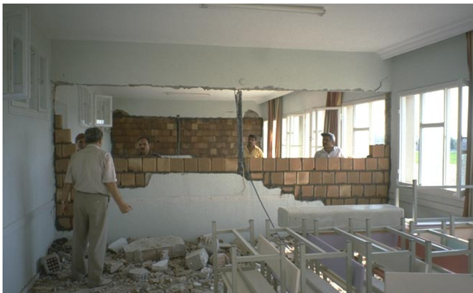
Fig. 23 School buildings west of Ceyhan: Reconstruction of a destroyed masonry infill wall
