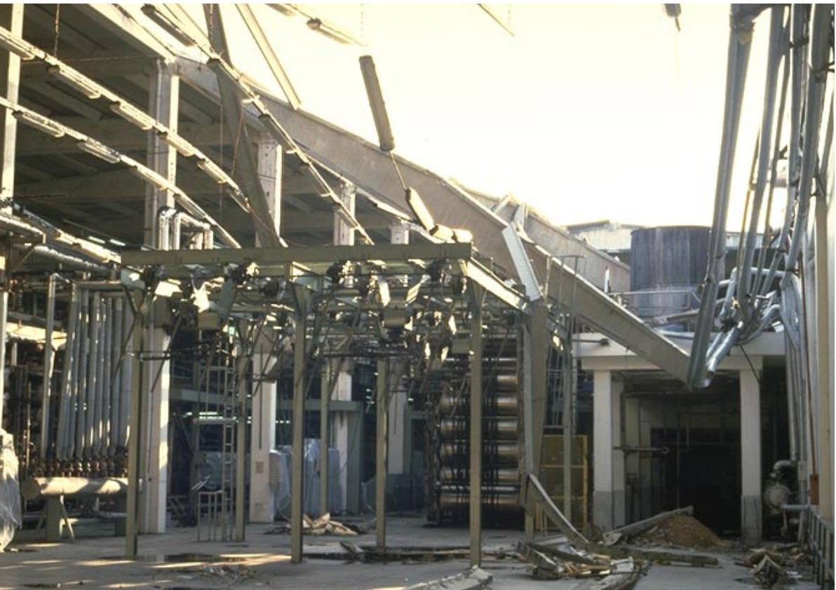
Fig. 27 The collapsed roof destroyed one of two dye work production lines (damage grade 4)
