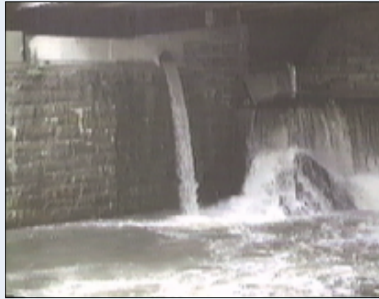
Untreated sewage flows from a CSO outfall directly into the Blackstone River. A 20-year project is underway to eliminate such discharges. Photo: Narragansett Bay Commission
