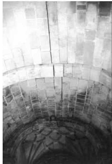
Figure 6 : Grietas in the vault
