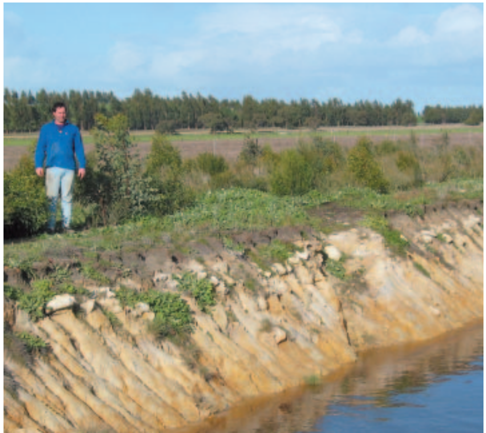
Above: Deep drains have relieved the impact of rising water tables but introduced soil management challenges.
