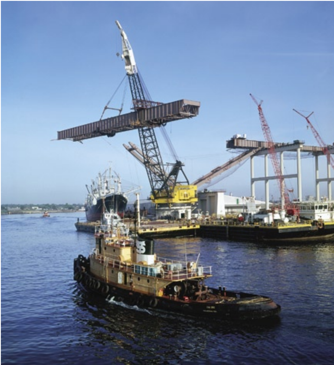
Heavy lifting: A steel girder for the approach span is lifted into position in June 1971. (Photo: TxDOT)
