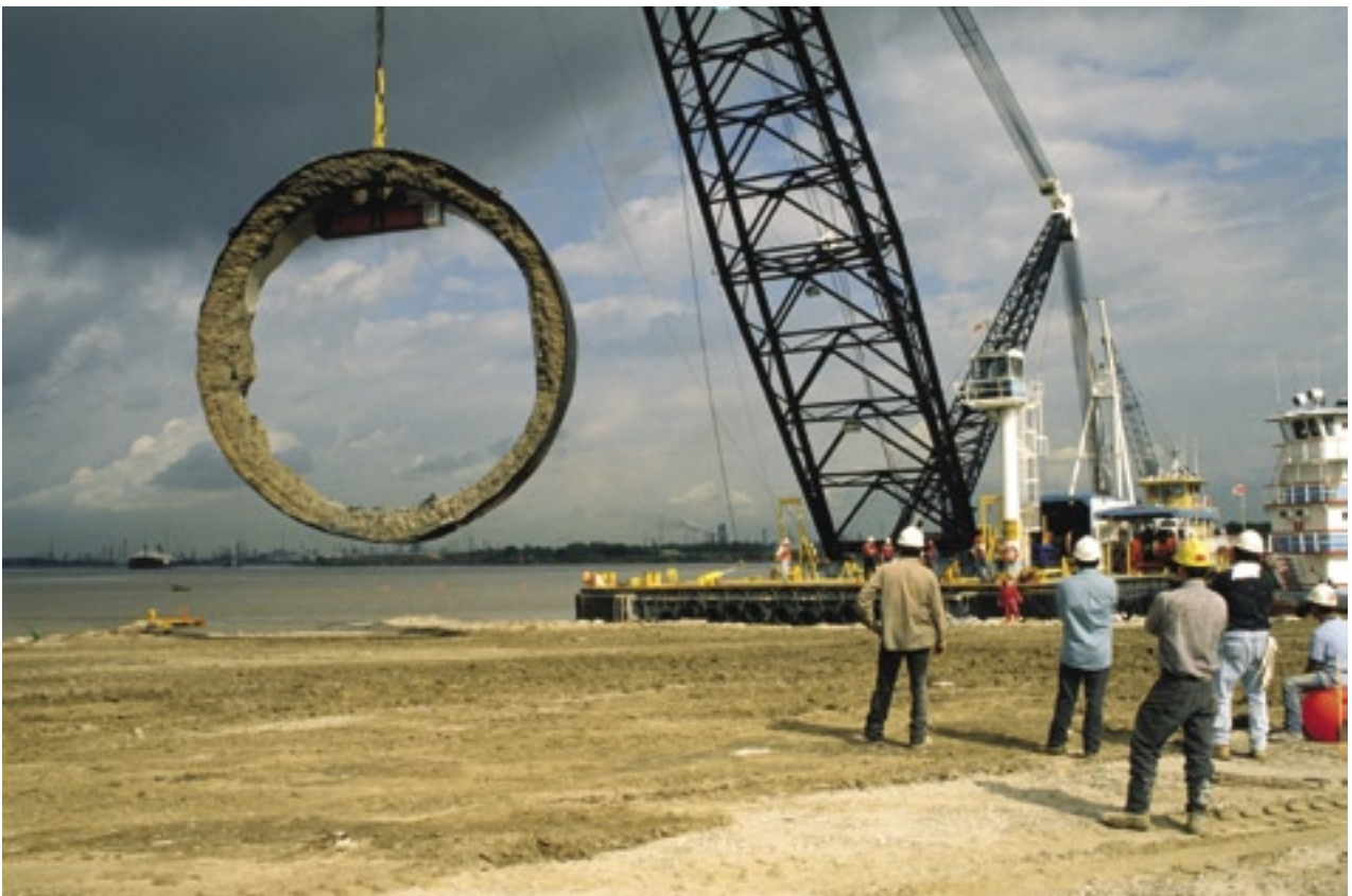
Tunnel removal, 1998: Because of a planned deepening of the Houston Ship Channel, the tunnel needed to be removed soon after the bridge was opened. Initial plans to cut the tunnel into sections and then transport the sections to an artificial reef area in the Gulf of Mexico did not move forward. In a second round of bidding, the bridge contractor submitted the winning bid with a plan to slice the tunnel into sections and recycle the material. The removal of the Baytown Tunnel appears to be the first removal of an underwater vehicular tunnel in the United States. (Photos: TxDOT)
