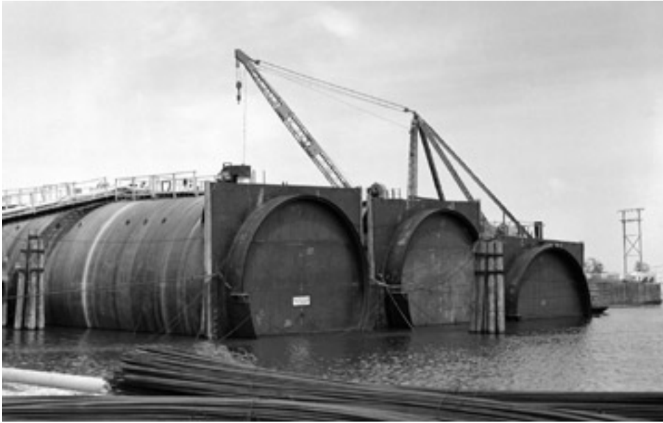
Building the Baytown Tunnel: The underwater tunnel sections were fabricated at a steel mill in Orange, Texas. With the ends sealed, the floating tubes were towed 125 miles (200 km) along the intracoastal waterway and the Houston Ship Channel to the tunnel site. (Photo: TxDOT)
