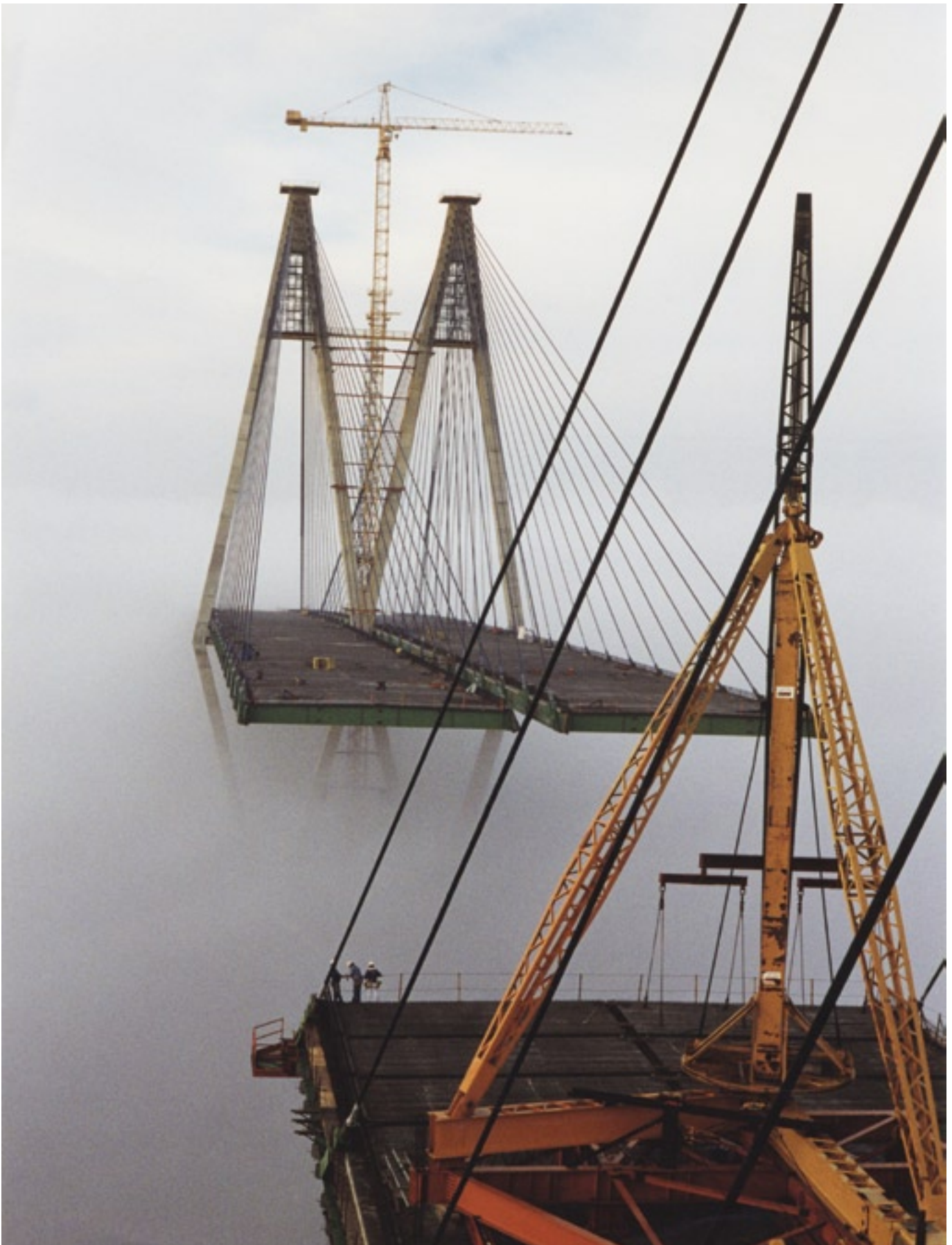
Emerging from the fog: This view shows the main bridge deck nearing completion in 1995. Around the time of this photo, the project schedule was also emerging from a fog, much to the relief of motorists. (Photo: Williams Brothers Construction)
