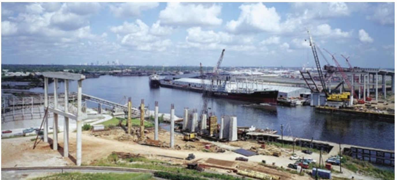
Approach construction: This June 1971 view looking northeast shows the first “V” strut being positioned. (Photo: TxDOT)
