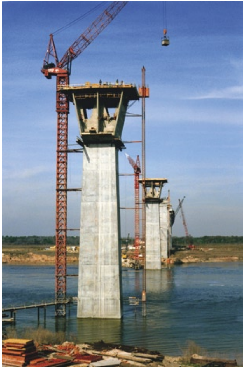
Pier construction: This 1980 photograph shows the piers for the main span taking shape. The reason for calling this type of bridge a concrete box girder can be seen in this photo. The "box" is the cross section of the bridge's main span, visible at the top of the pier. In this bridge the box actually has the shape of a trapezoid. (Photo: North Texas Turnpike Authority)
