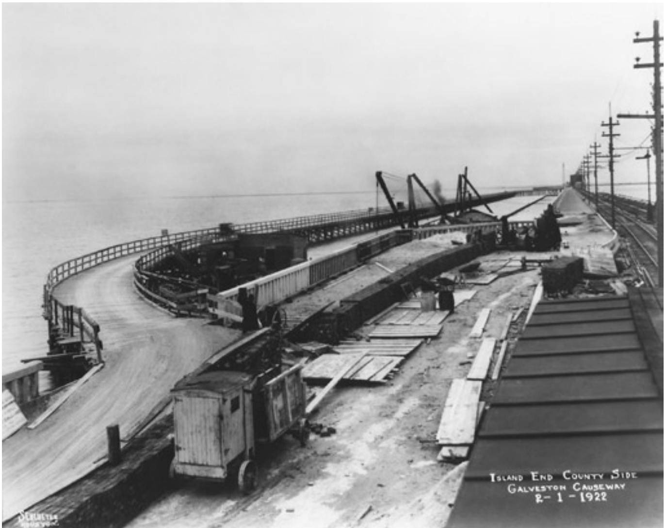
Repairing the damage from the 1915 hurricane: The bridge structure itself survived the hurricane with virtually no damage, but the earthfill sections leading to the bridge were washed away. Temporary wooden rail trestles from the shorelines to the bridge were immediately constructed to restore rail service. Permanent repairs extended the concrete bridge structure to replace the earthfill sections. This 1922 photograph shows the repair work nearing completion. Vehicular traffic used a temporary wooden bridge which connected to the unharmed 1912 structure in the distance. (Photo: Rosenberg Library G-18221FF2.12#7, Galveston)
