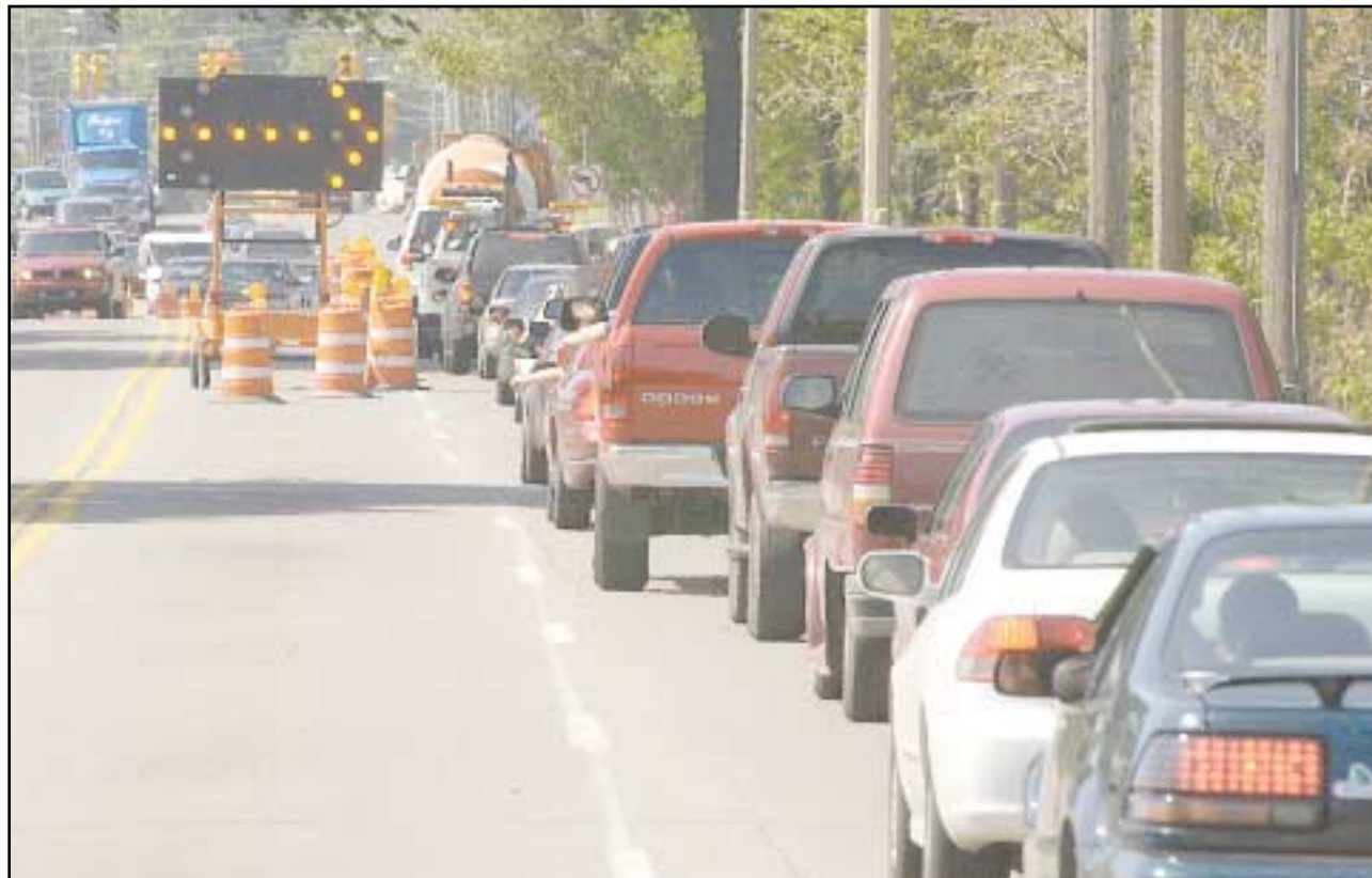
JAM: Traffic on River Avenue backs up on Monday afternoon at the intersection of River and Howard avenues as BPW crews worked to repair a water main that was damaged Sunday.
