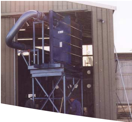
New plate heat exchanger condenser and stand
