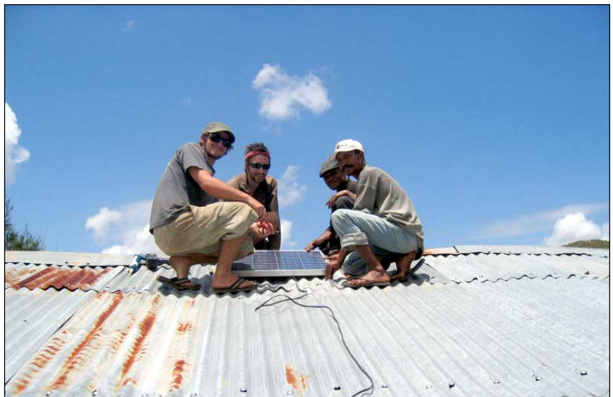
Installing a solar panel on a health clinic in the isolated enclave of Oecussi. This panel was capable of running six compact fluoros for up to four hours per night.
