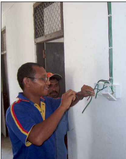
Local people were trained and assisted with the installation of all the systems.
