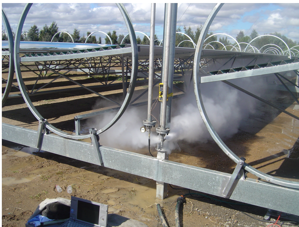
Fig. 4. The array venting steam for the first time on August 19.
