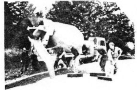
Fig. 4 Pouring and laying the concrete at ground level on the pneumatic from still deflated.
