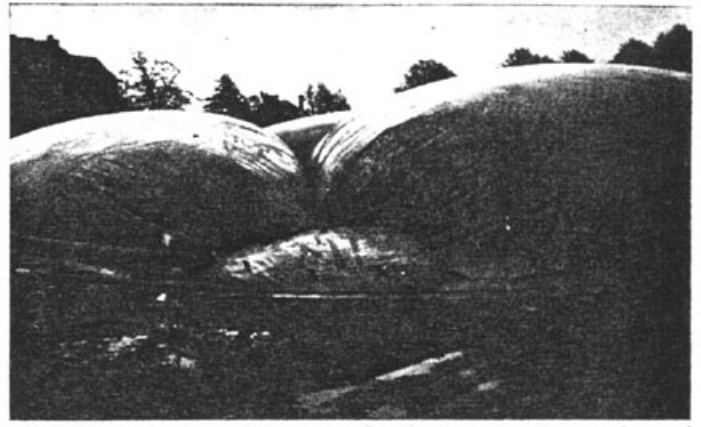
The inflation membrane being test inflated prior to setting out the steel reinforcement. The rainwater held in the folds of the membrane was much more than realised, which eventually gave unsuspecting sitemen a heavy baptism.
