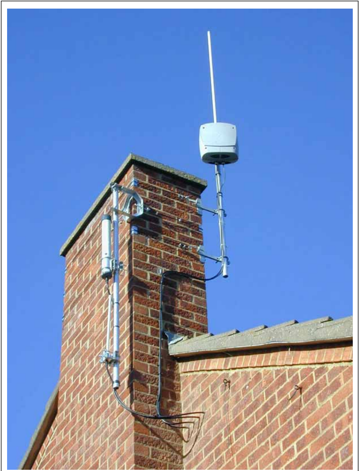
Figure 2-10: Histon Wi-Fi hotspot co-installed with CBL Outdoor Unit
