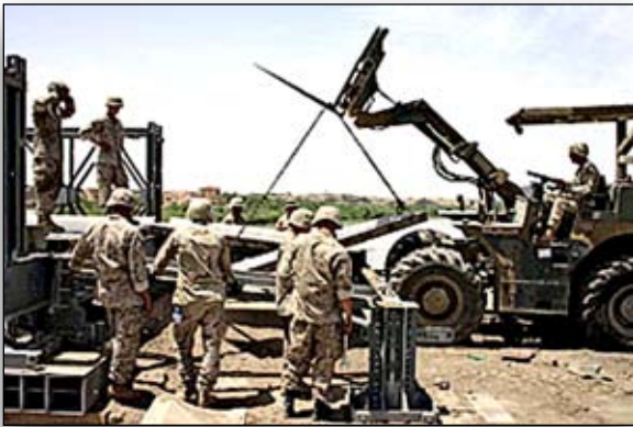
Building bridges may not have been what the soldiers of the U.S. Army's 216th Engineer Battalion expected to be doing in Iraq. But with the help of Marines from 6th Engineer Support Battalion, they participated in the $4 million Tikrit Bridge rebuilding project in Tikrit, Iraq during 2004. (Photo by Army SPC Joe Alger)
