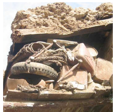
Fig 28: Very poor building, Bedadi village.
