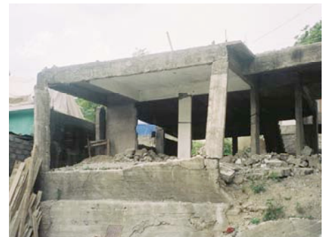
Fig 24: This roof stayed up, unlike many others. Chella-Bandi, Muzaffarabad.
