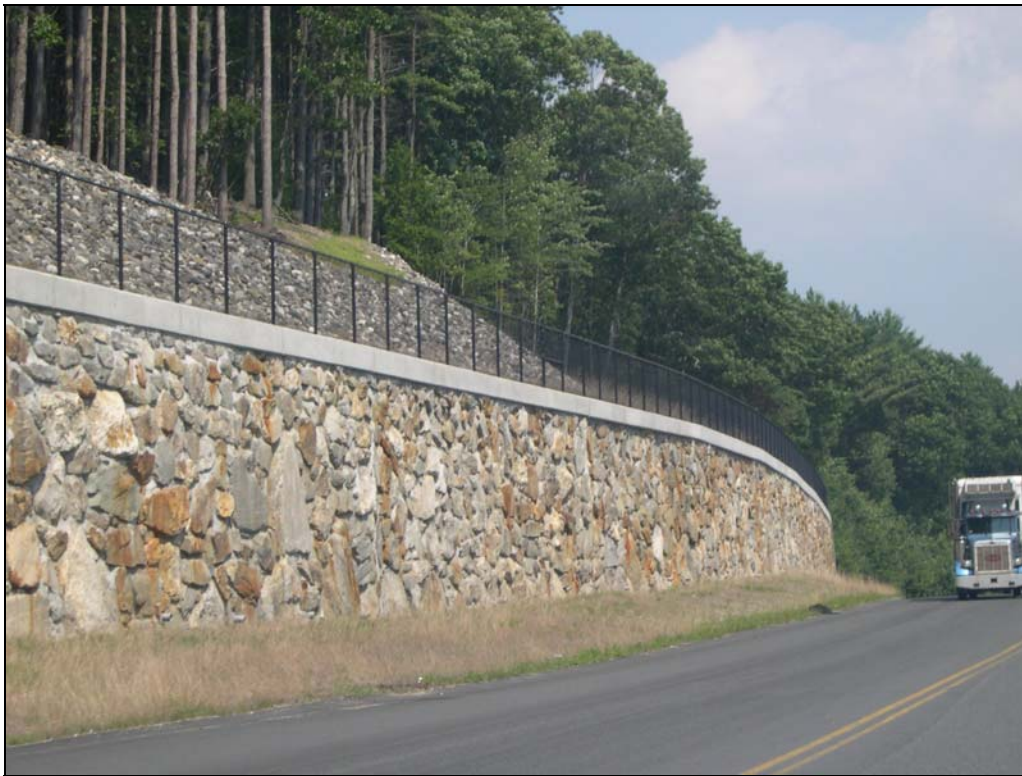
New retaining walls along the relocated Route 2 at the Erving Paper Mill were built using stone excavated during construction
