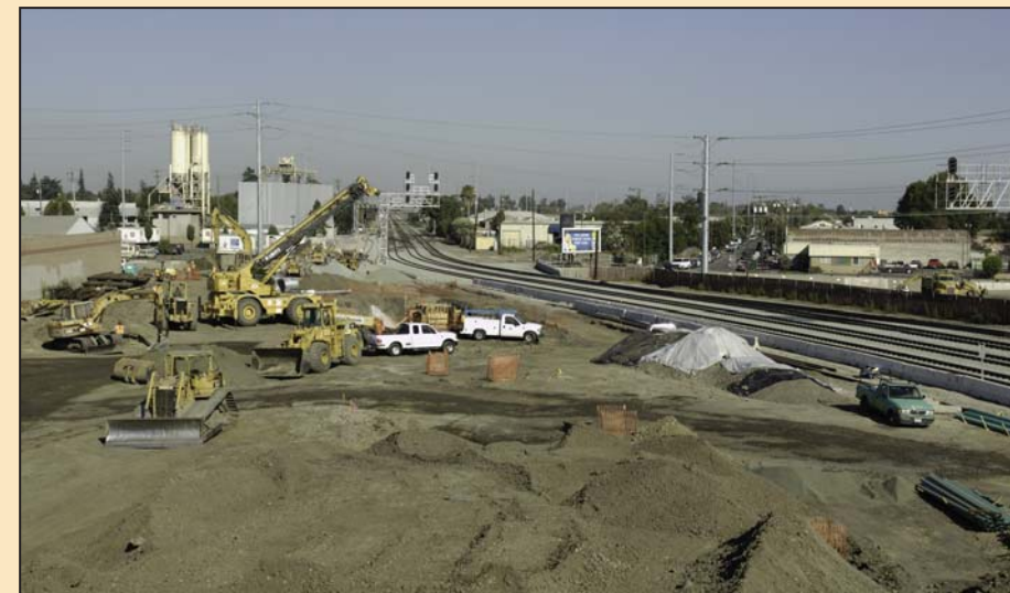
Shielded by a community wall (left), work has been under way since 2005 at the CEMOF site in San Jose, which is bounded by Coleman, Lenzen and Stockton avenues and by West Taylor Street on the south.
