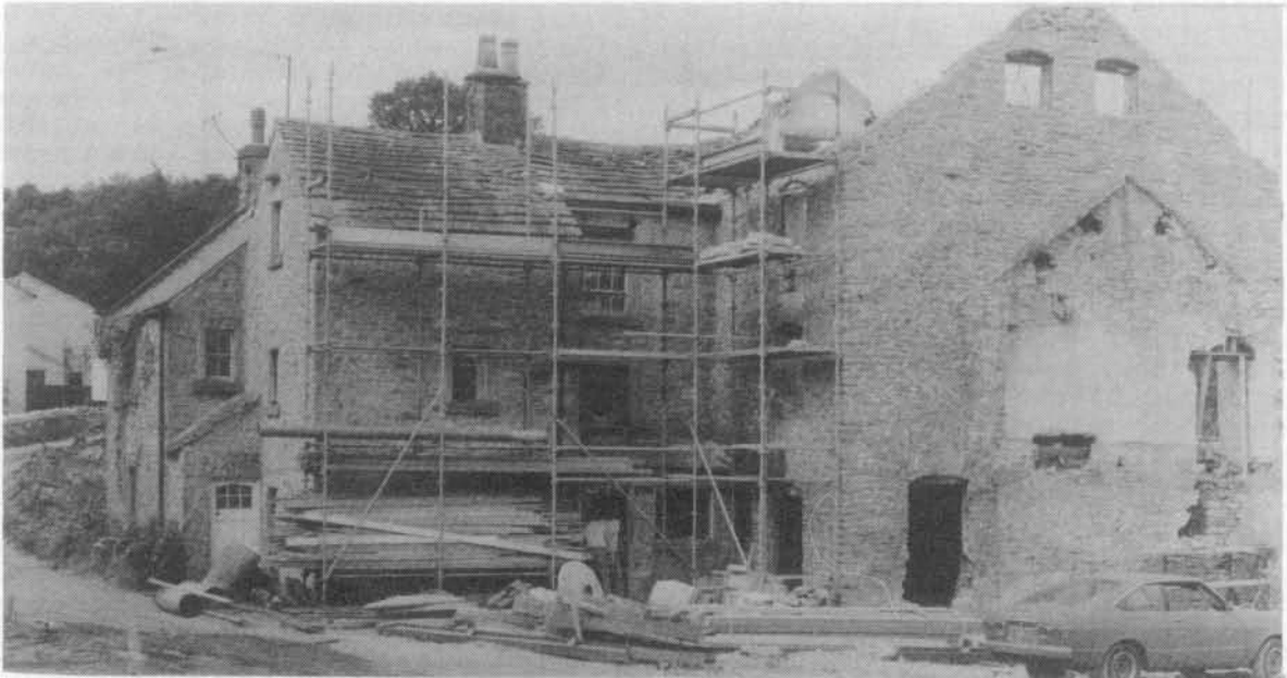
View from the opposing side, the mill building is to the right, following demolition of a later extension.
