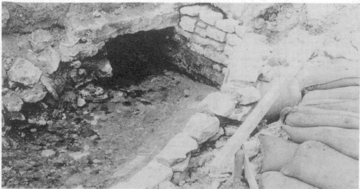
Unroofed section of a sough, which passes under the southerly, lower and older pond. The water in it flows from Brightside Sough, though its tail is today higher up the valley.
