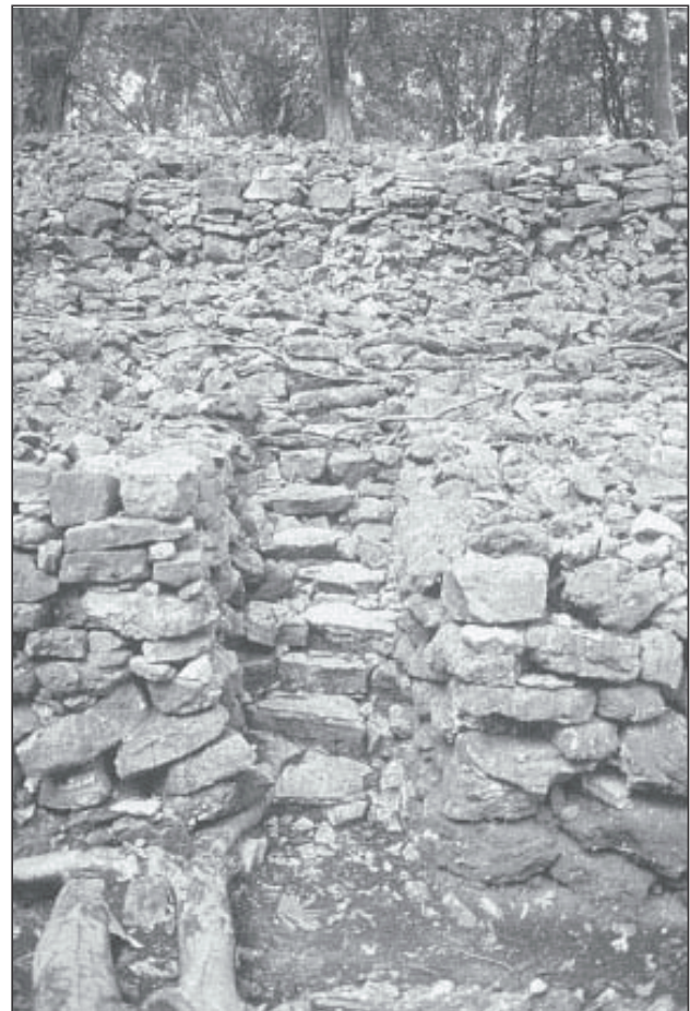
Figure 7 The passage between construction bins after restoration. Note the coarse stairs in the passage (the stairs are not restored).
