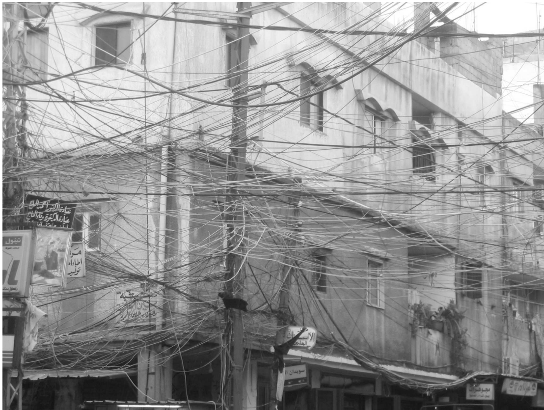
Criss-crossing cables in Nahr al-Bared refugee camp, March 2005, © AI
