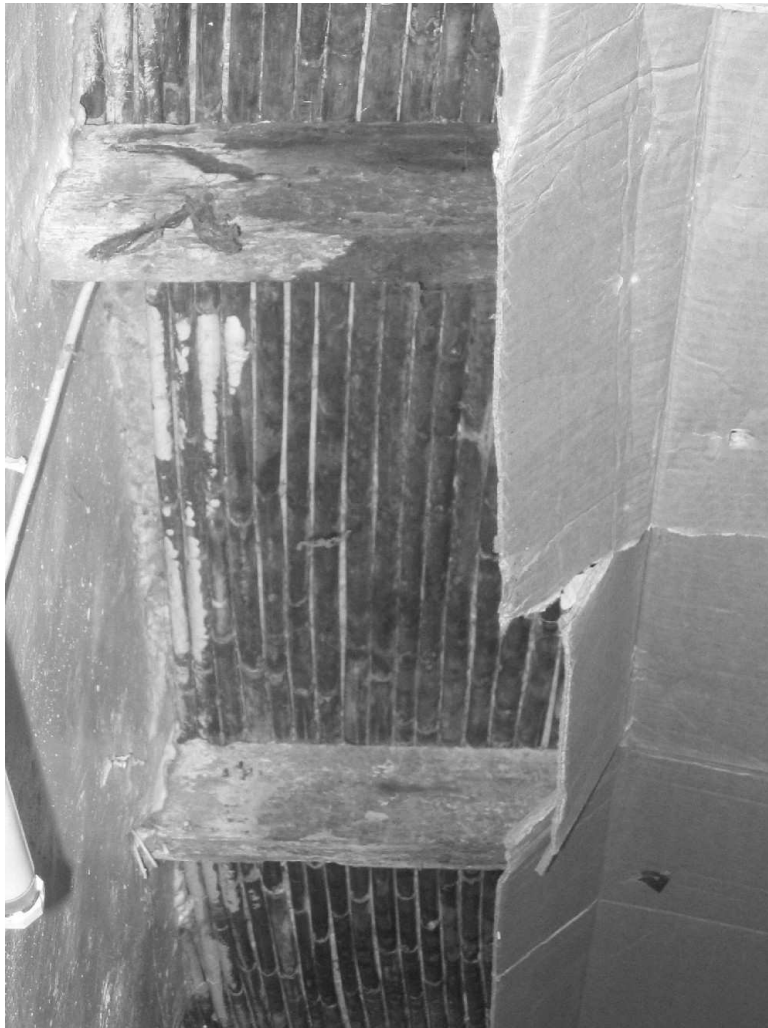
Roof coverings made of wood and sticks and cardboard in el-Maachouk camp, March 2005, © AI
