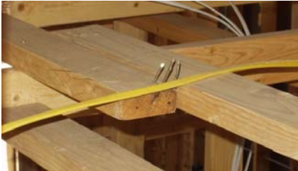
Nails come dangerously close to electrical wiring in this attic, posing a potential safety hazard
