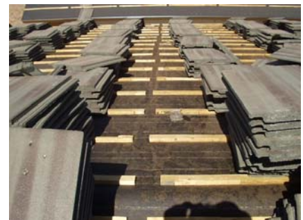
Roof battens should be evenly spaced, allowing for proper drainage and preventing future damage.
