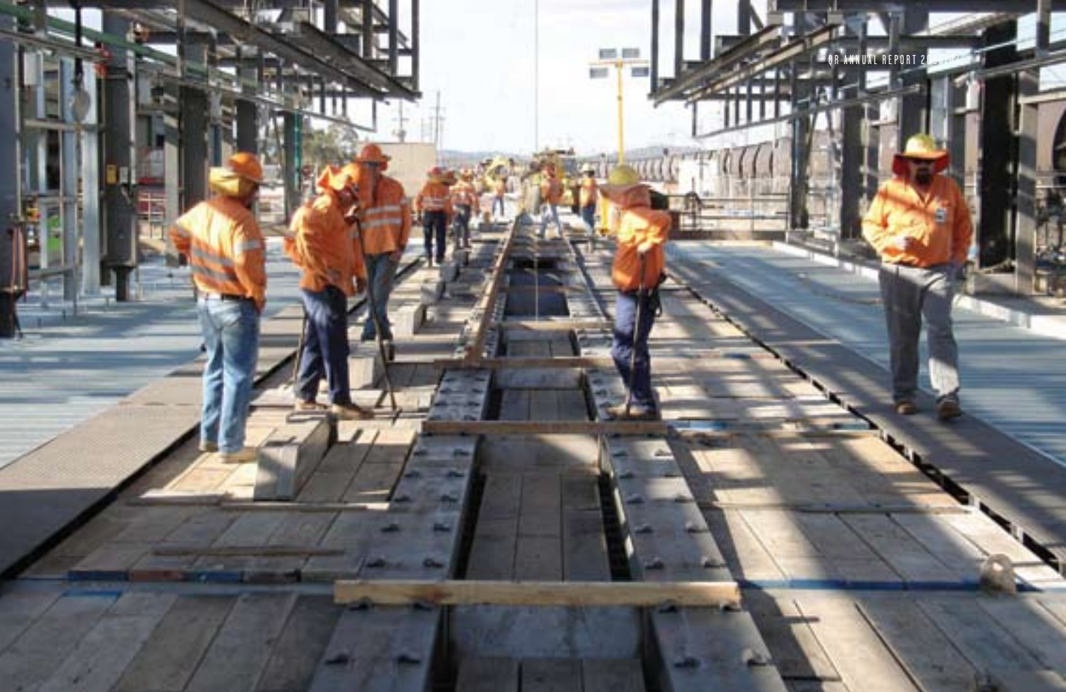
Construction of RG Tanna third unloading station underway by QR infrastructure crew.
