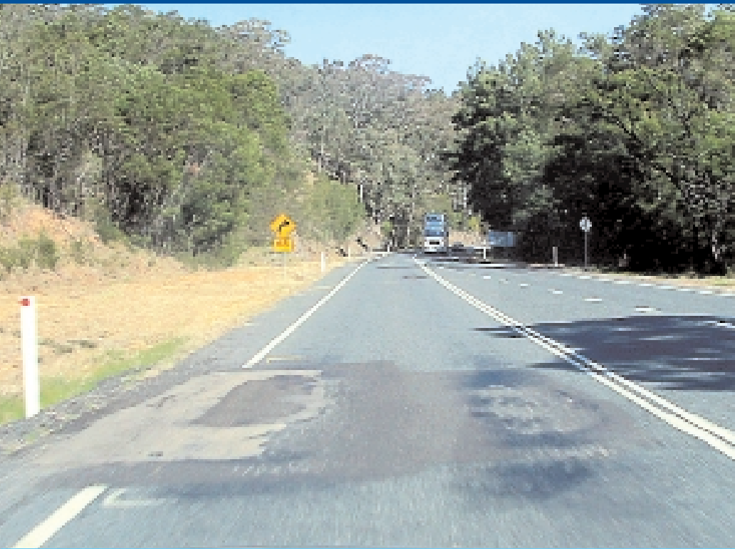
The patchy surface of the Kings Highway 8km from Batemans Bay
