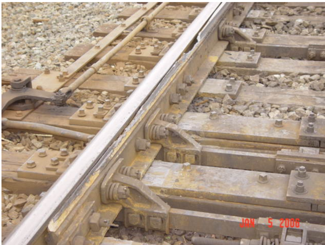
Figure 2. Looking north at the reverse, or left, switch point, which was the point of derailment.
