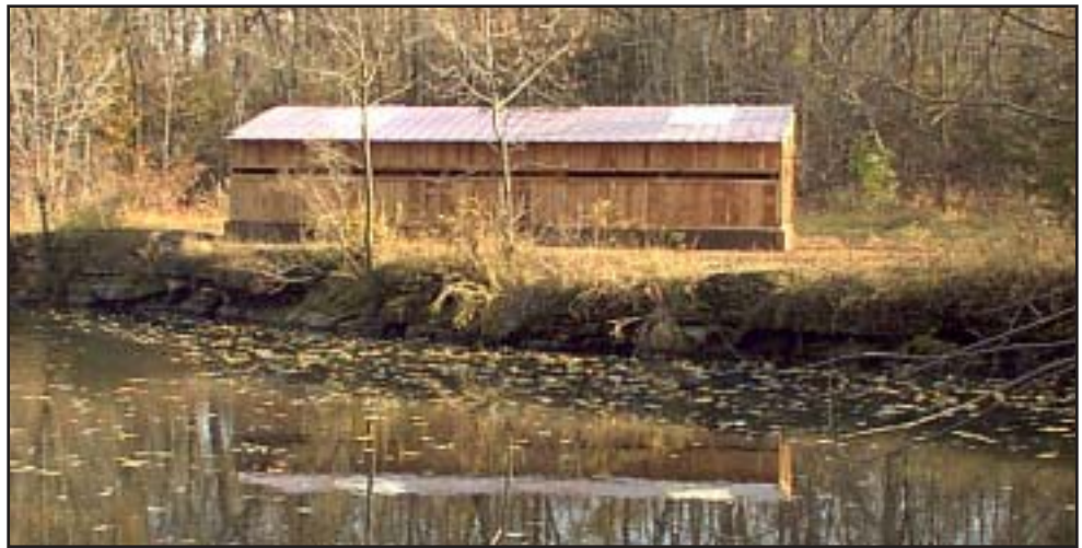
Above: The bird blind at Jakway Park is back in place after having been washed off its foundation by flood waters in May, 2004.
