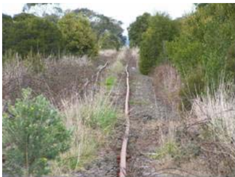
Figure 9-4: Km 70.7: Formation Failure
