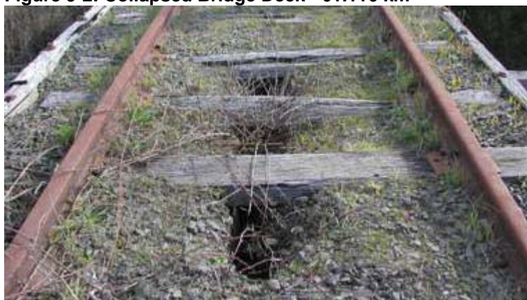
Figure 9-2: Collapsed Bridge Deck - 61.116 km
