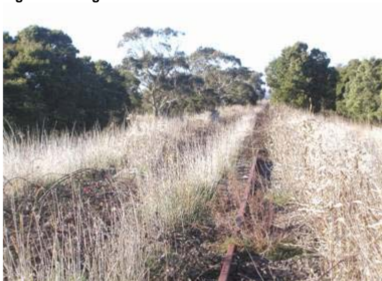
Figure 5-1: Vegetation on track
