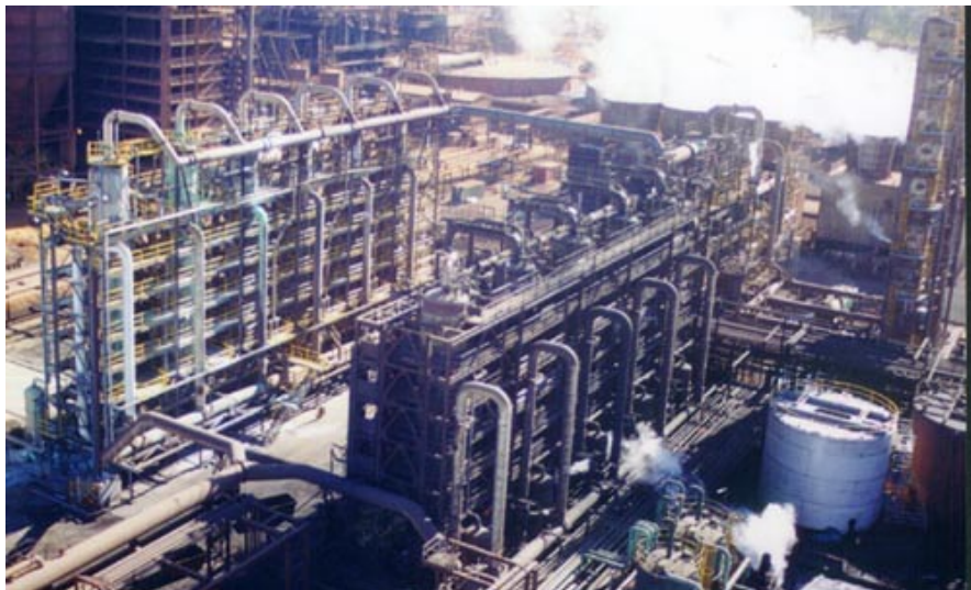
Figure 4. Steam stripping columns used for ammonia and carbon dioxide recovery
