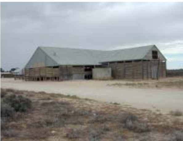
Figure 5.4 The Woolroom at right of image was underpinned during 1990s works. Compare to Figure 2.7.
