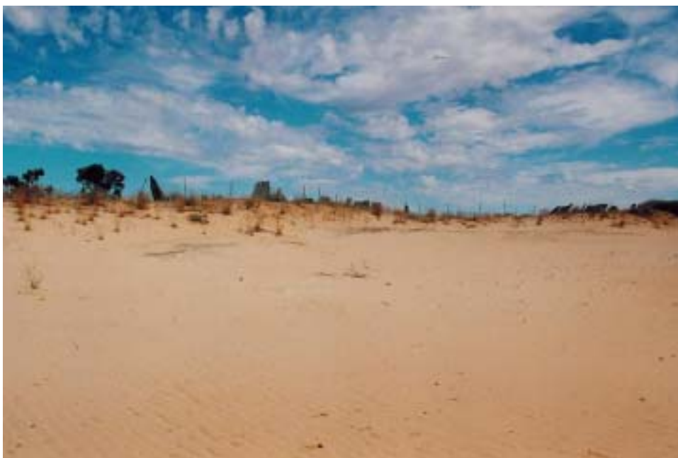
Figure 4.4 The dilapidated state of erosion control fences at MA 109 have resulted in the site again being subject to rapid erosion.
