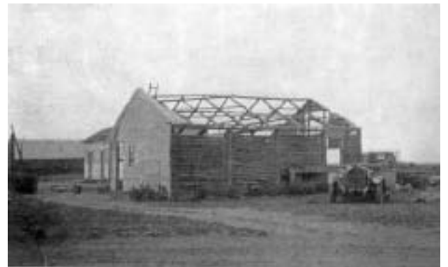
Figure 5.14 Shearers Cookhouse during demolition in 1954. (Note current Shearers Quarters in the background) (Barnes Family Collection).
