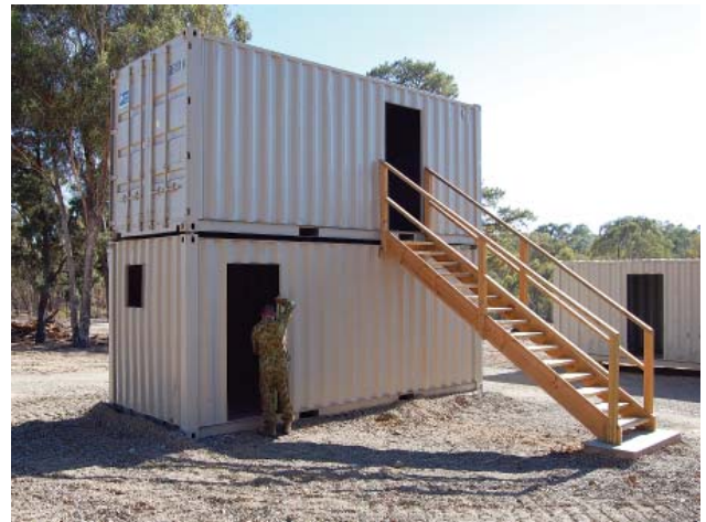
Work proceeds on shipping containers that form part of the Urban Operation Training Facility at Puckapunyal, Victoria.
