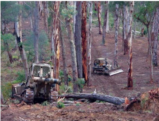
Dozers clearing scrub during the construction of a containment line in preparation for the Victorian bushfire season.
