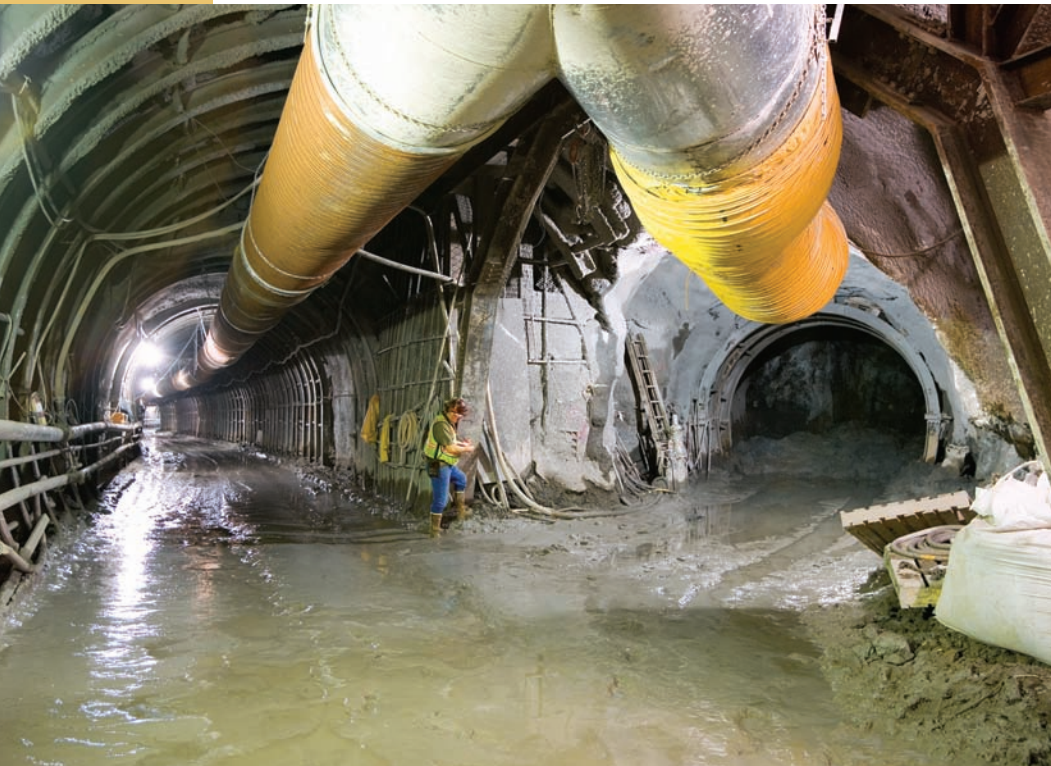
The "access" tunnel on the left will provide a permanent entry for the "bypass" tunnel on the right. The bypass tunnel will connect to the existing tunnel when completed in 2007.
