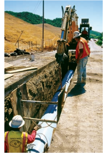
Workers lay a 36-inch diameter pipe during construction of the Southern Loop Pipeline along Crow Canyon Road in Castro Valley.
