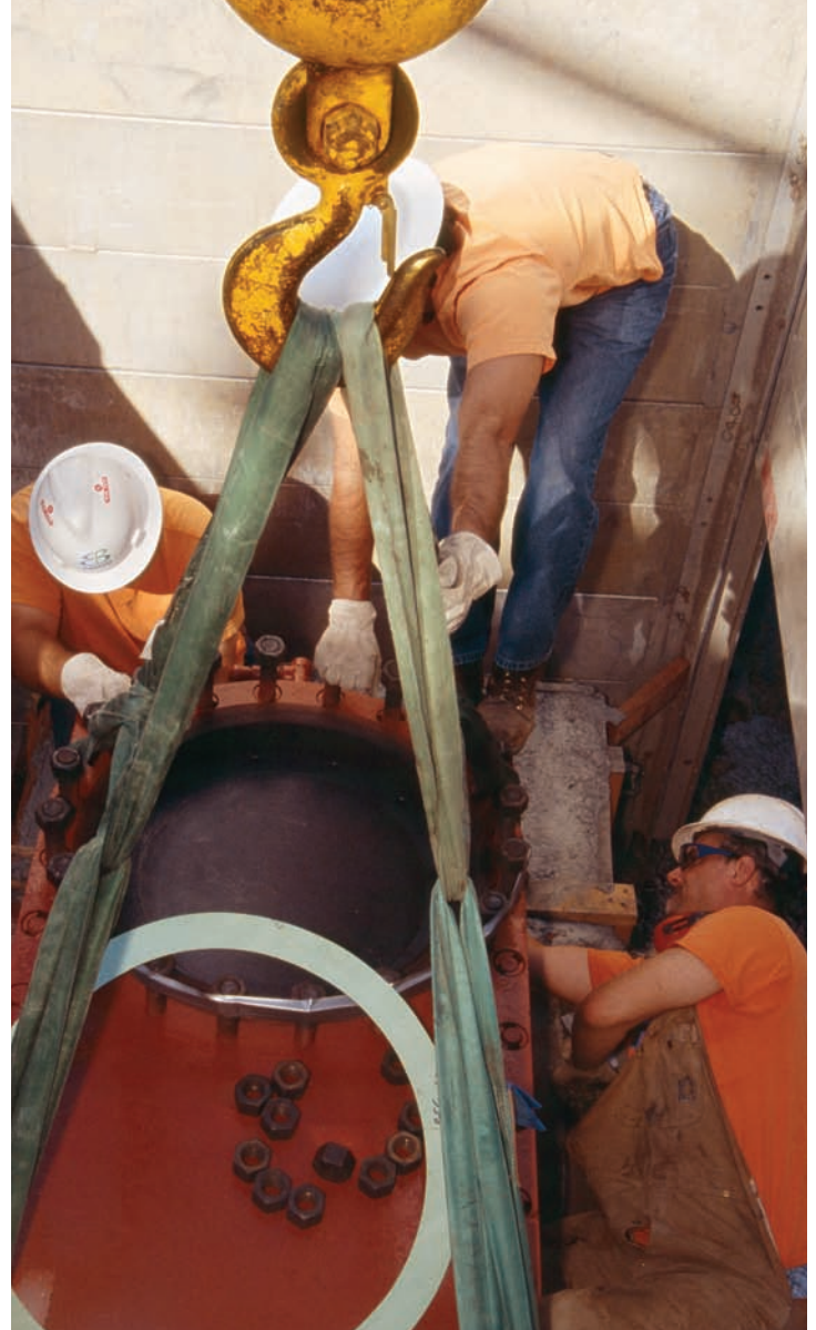
Workers install a 42-inch manifold to protect critical pipelines prone to landslide damage.
