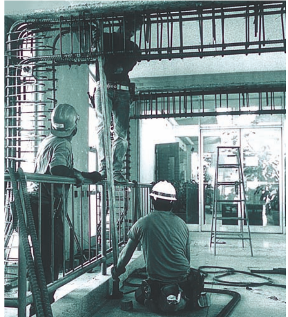
Workers install a seismic retrofit to strengthen the filter gallery at one of five upgraded water treatment plants.
