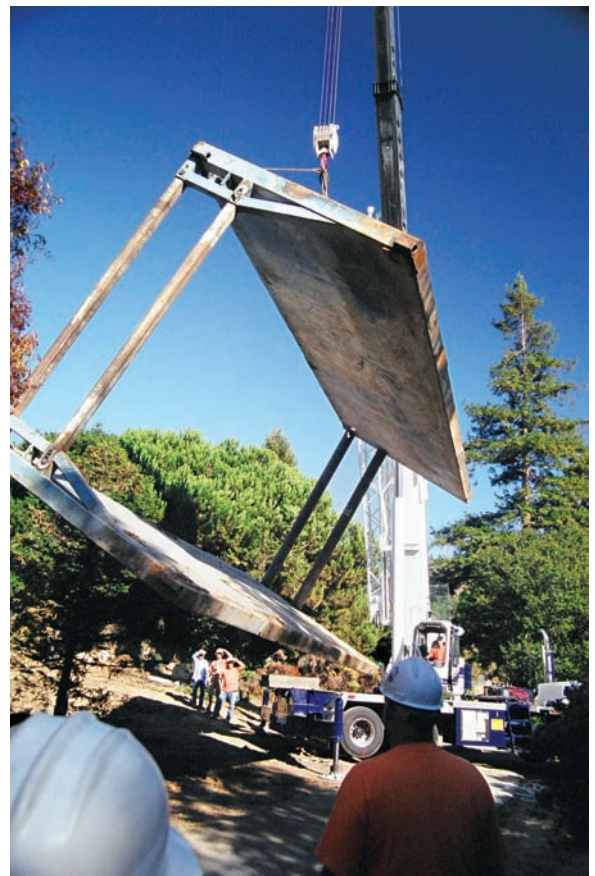
Crane lowering a shoring box (above) to reinforce the sides of a major transmission pipeline crossing a fault at Lake Temescal. With the shoring box in place (left), work to prevent water loss at this fault crossing location was completed.
