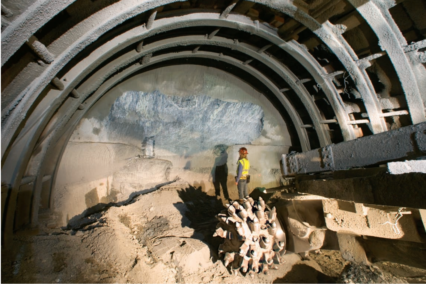
The tunnel excavation (above) is inspected continuously for changes in geology and to assure compliance with design requirements. The roadheader mining machine (below) grinds the rock face into fine gravel as it excavates.
