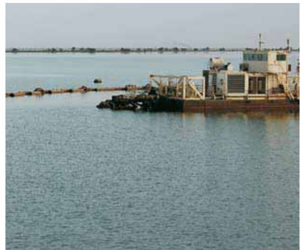
At the Roseires dam reservoir, a dredger is continuously used to remove sediment from the electric turbine water inlets. Soil washed from the Ethiopian highlands is the main source of the sediment
