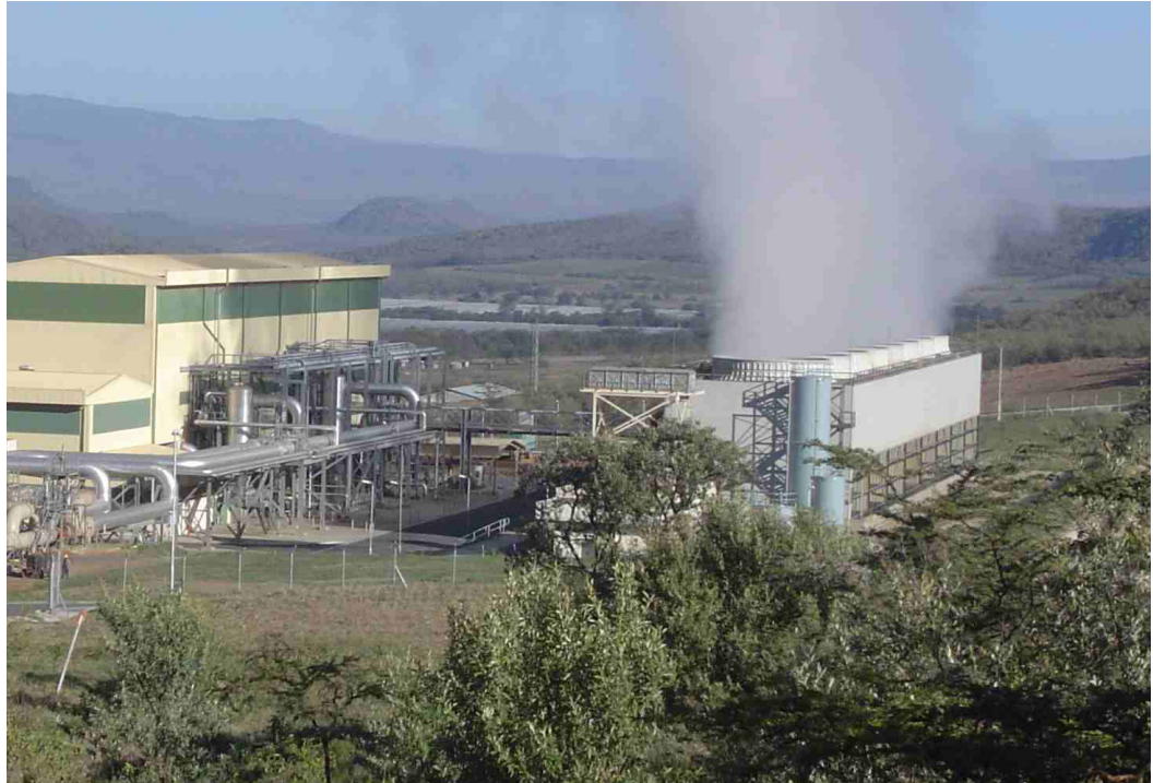
Figure 3.6: A Mechanical Draft Cooling Tower.
