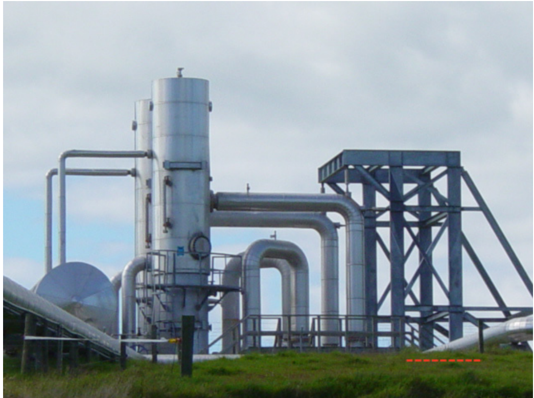
Figure 3.8: Steam Separators and Brine Accumulators.
