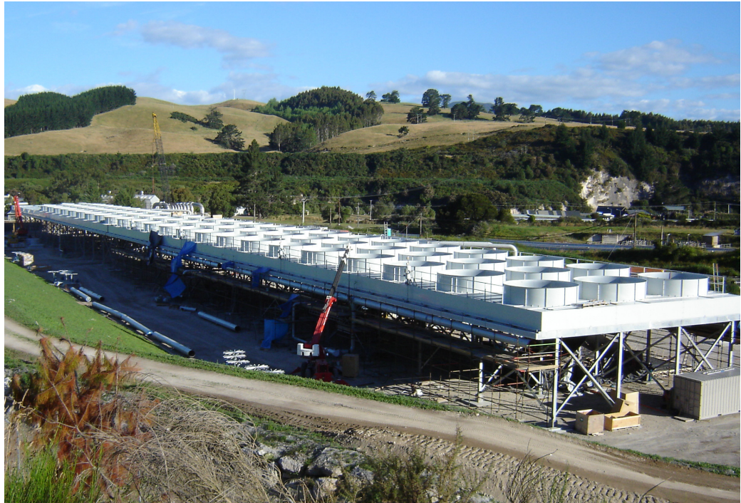
Figure 3.5: Air Cooled Condensers.
